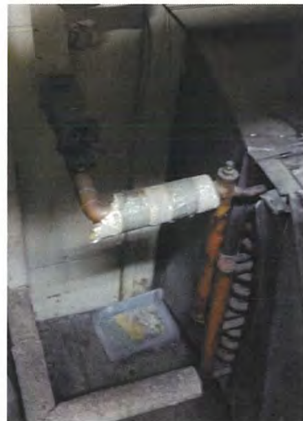
Photograph #4 – Zone #2 Heating Water Coil
