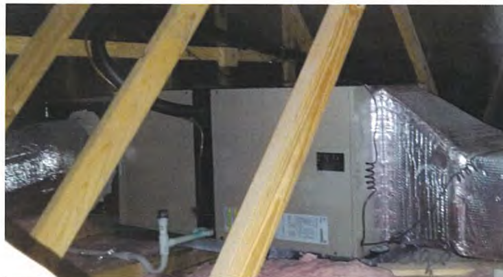
Photograph #5 – Zone #3 Air Handling Unit
