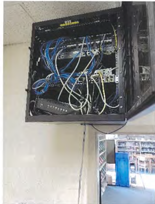
Photograph #18 – Wall Mounted Data Rack
