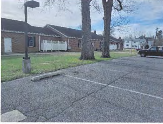
Photograph #15 – Pole Mounted Parking Lot Light Fixture
