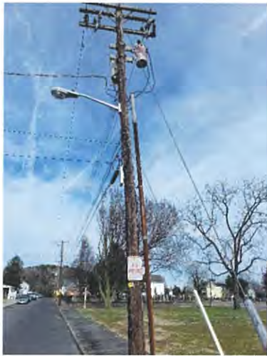
Photograph #9 – Pole Mounted Utility Transformers
