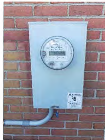
Photograph #10 – Utility Meter Installed on Exterior Wall of Boiler Room
