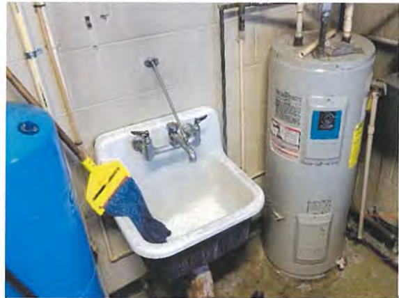
Photograph #6 – Hot water heater, associated expansion tank and service sink
