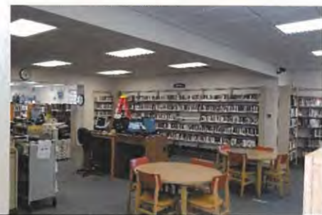
Photograph #12 – Recessed 2'x4' fixture
