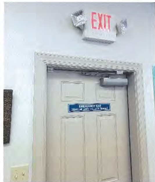
Photograph #14 – Typical Emergency Light Fixture
