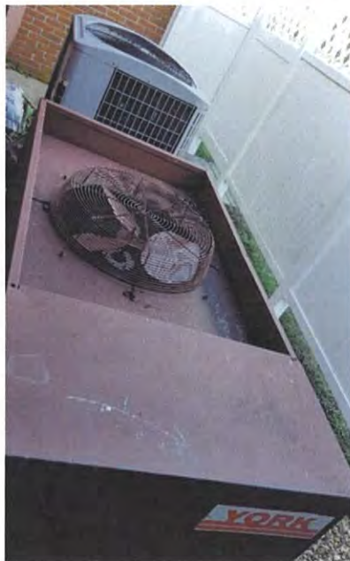
Photograph #3 – Outdoor Condensing Unit
