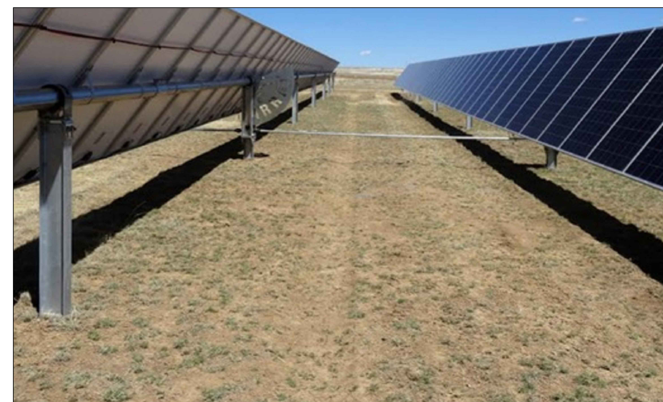
3 SIMILAR PV ARRAY
