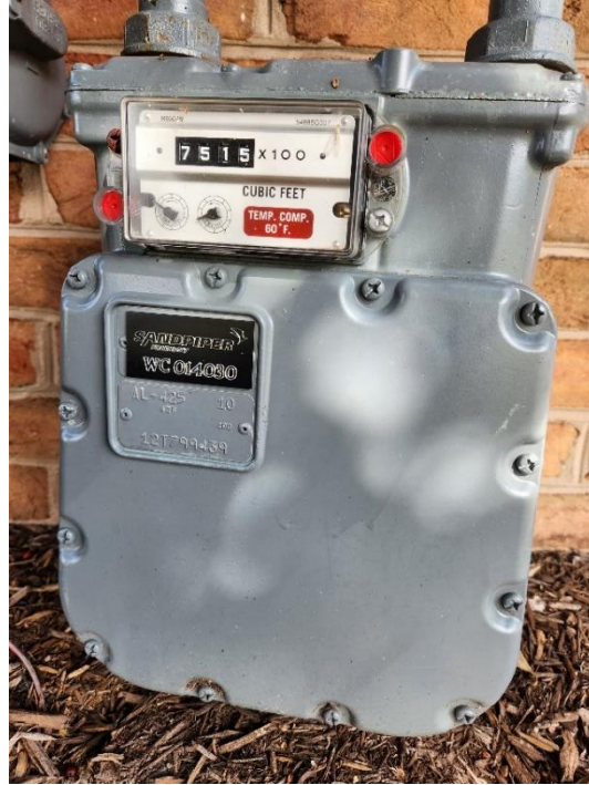
Photograph #28 – Propane Gas Service on Front of Building
