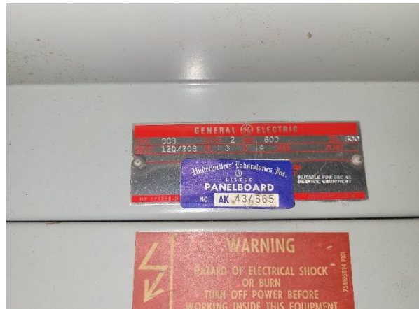
Photograph #34 – Panelboard SES 1
