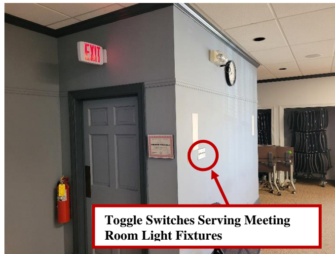
Photograph #45 –Toggle Switches Serving Meeting Room Light Fixtures
