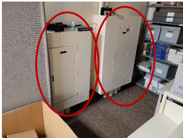
Photograph #33 – Distribution Panelboards SES 1 and SES 2
