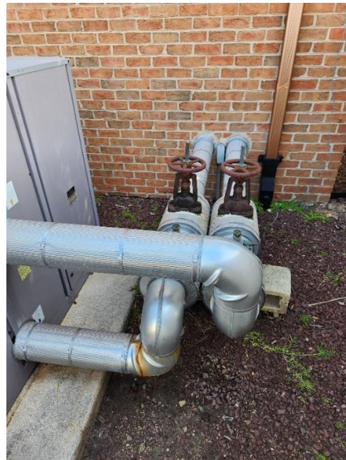
Photograph #17 – Exterior Chilled Water Piping
