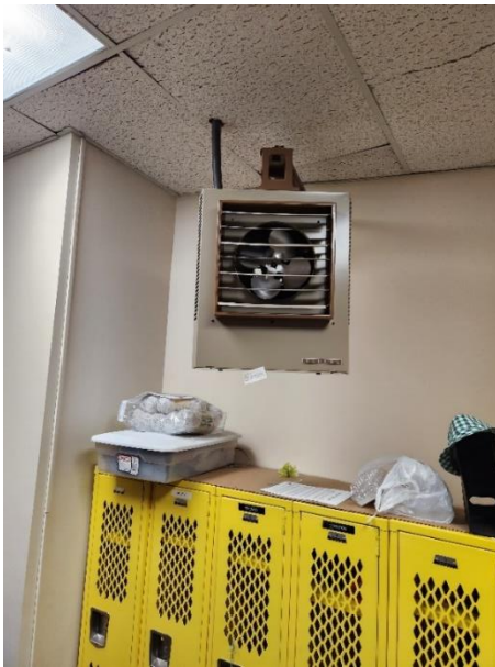
Photograph #22 – Typical Electric Horizontal Unit Heater
