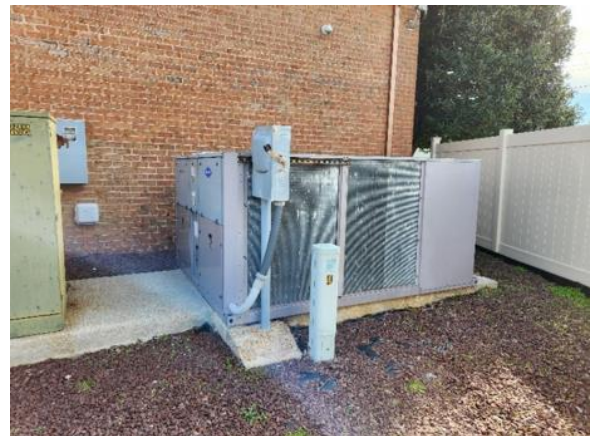
Photograph #13 – Air-Cooled Chiller
