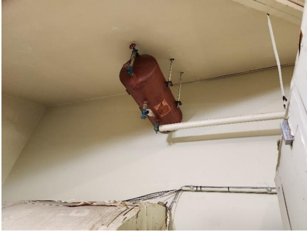
Photograph #10 – Chilled Water System Expansion Tank
