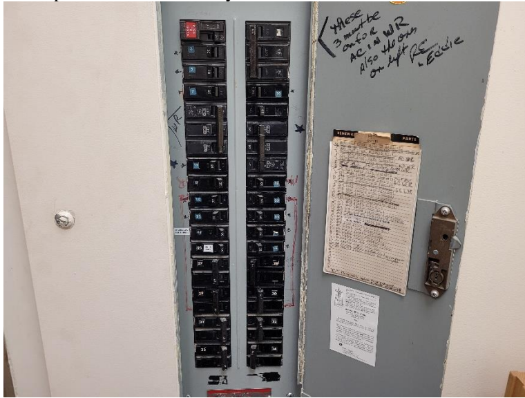
Photograph #35 – Panelboard H
