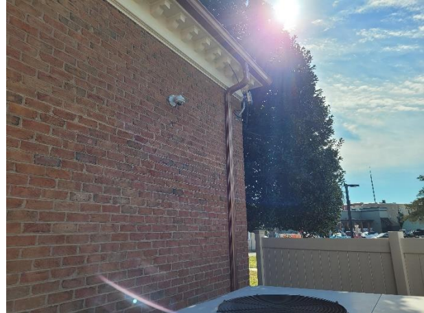
Photograph #58 – Exterior Video Surveillance Camera at Back Entrance
