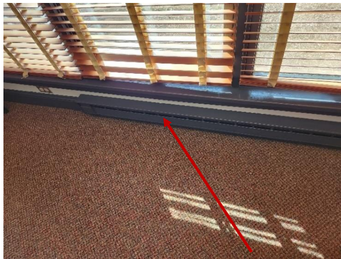
Photograph #24 – Typical Electric Baseboard Heat
