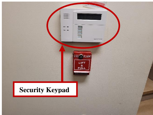
Photograph #55 – Security Keypad
