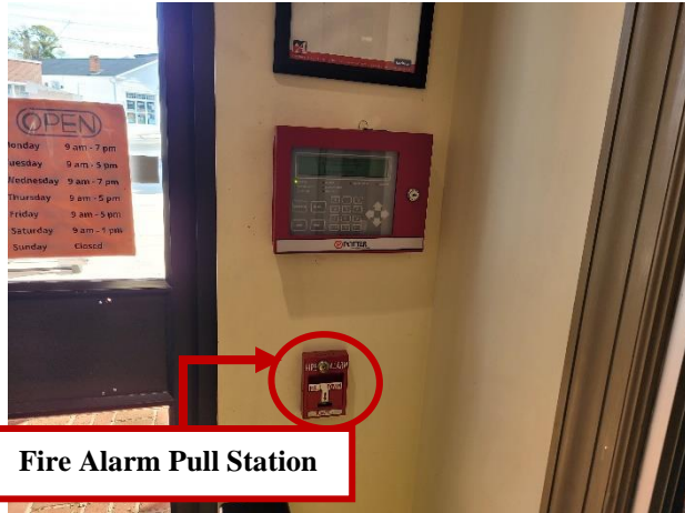
Photograph #53 – Fire Alarm Pull Station
