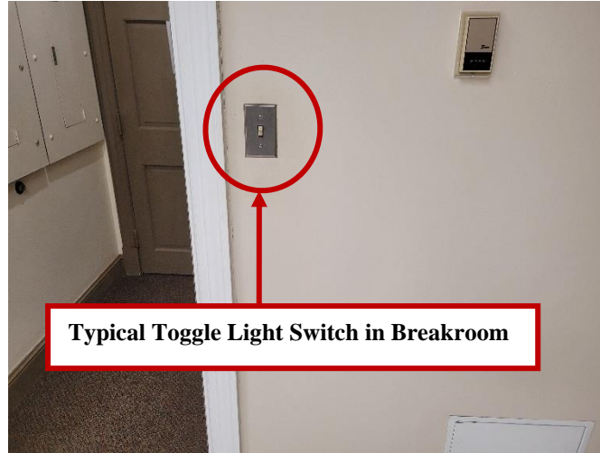
Photograph #44 – Typical Toggle Light Switch in Breakroom
