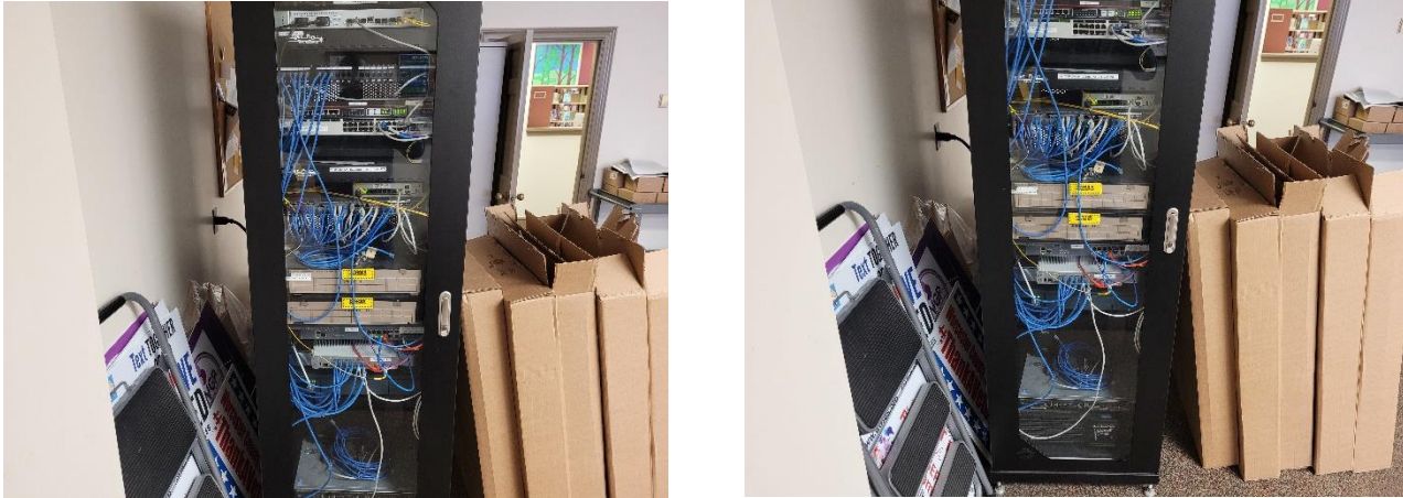
Photographs #59 and #60 – Servers/Network Switches
