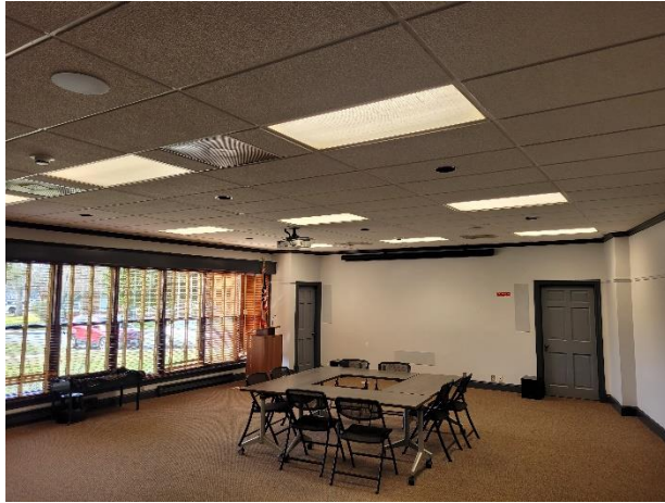
Photograph #42 – 2’x4’ Recessed Lighting Fixtures in Meeting Room
