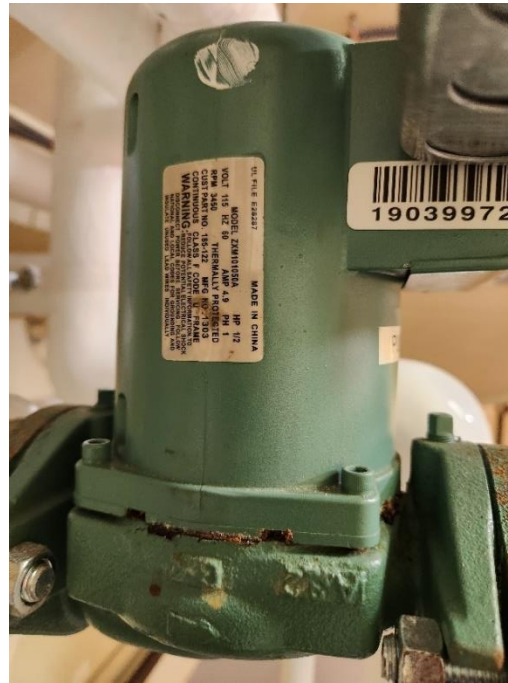
Photograph #2 – Boiler Primary Pump Motor Nameplate
