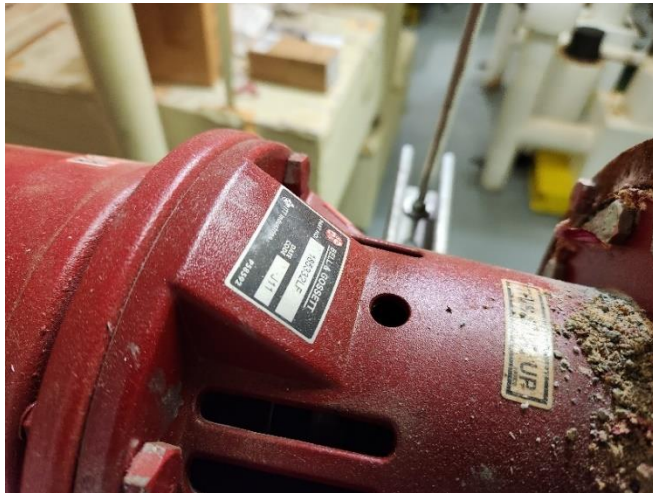
Photograph #3 – Heating System Secondary Pump Nameplate
