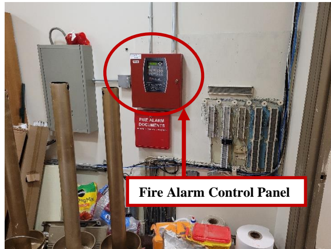
Photograph #52 - Fire Alarm Control Panel
