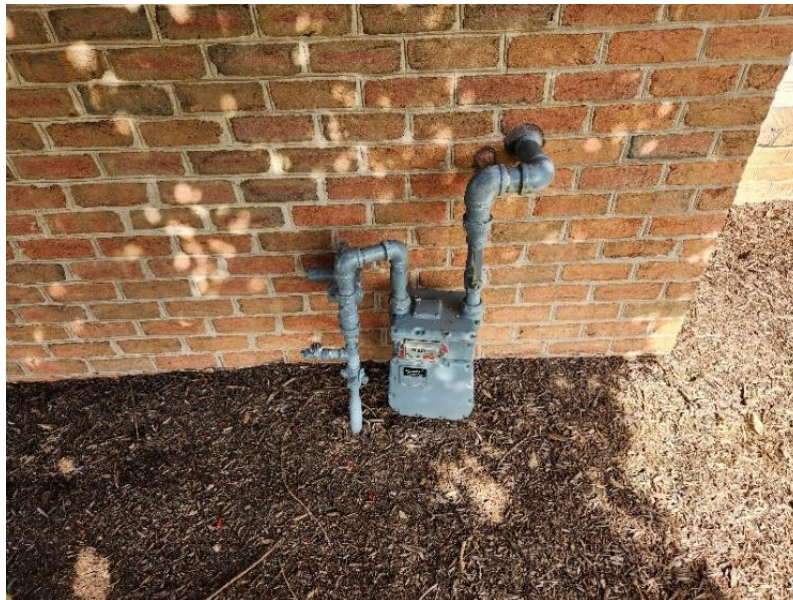
Photograph #9 – Central Propane Gas Service on Southwest Side of the Library
