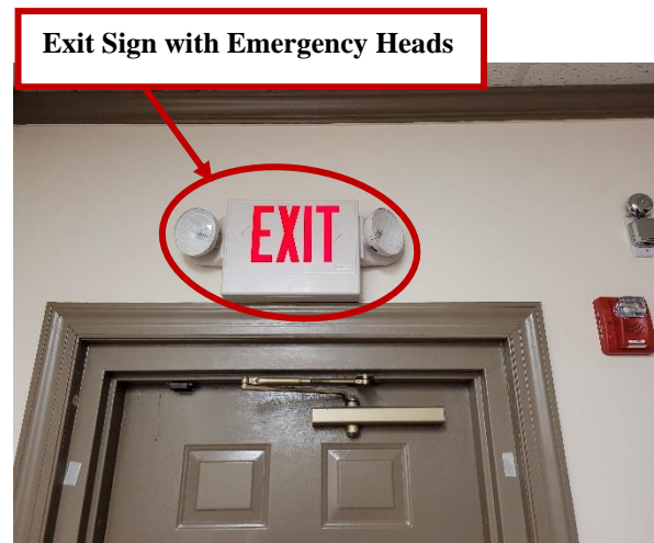
Photograph #47 – Exit Sign with Emergency Heads
