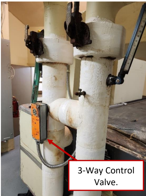
Photograph #16 – AHU #1 Chilled Water 3-Way Control Valve
