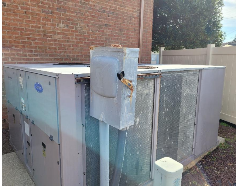
Photograph #40 - Disconnect Switch for chiller
