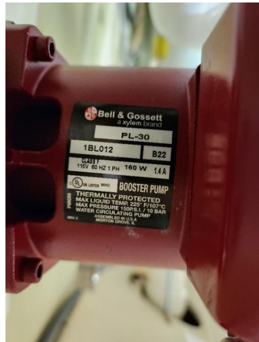
Photograph #4 – AHU #2 Heating Coil Pump Nameplate
