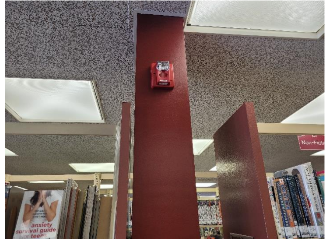
Photograph #54 – Fire Alarm Horn/Strobe
