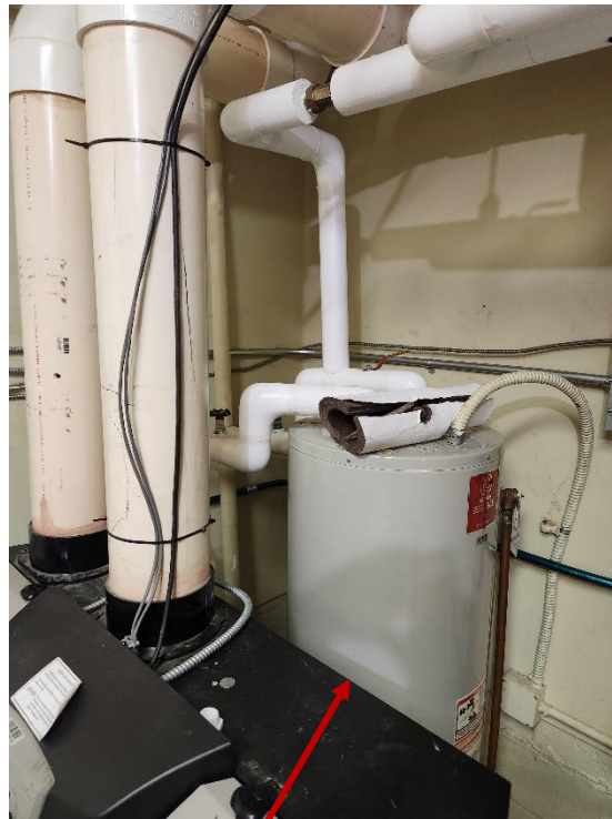
Photograph #27 – Electric Water Heater
