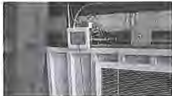
Photograph #3 – Existing Space Thermostats
