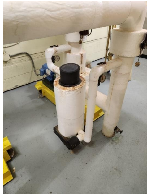
Photograph #11 – Chilled Water Chemical Feed Tank
