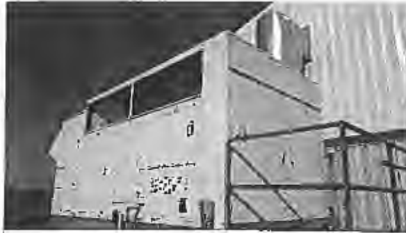
Photograph #1 – Existing RTU #1
