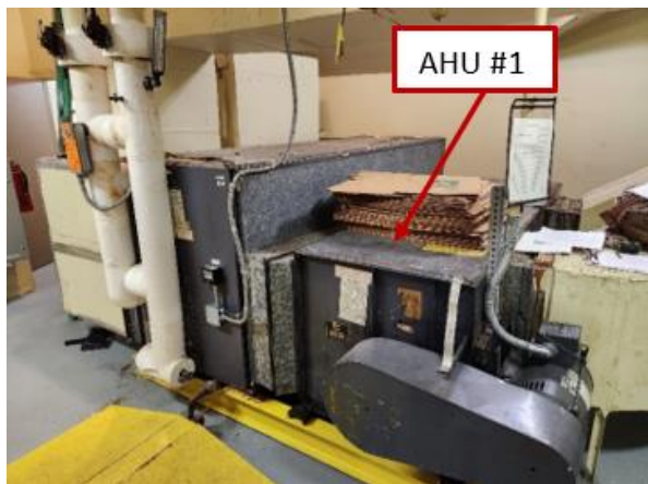
Photograph #18 – Air Handling Unit #1
