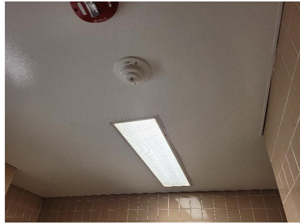
Photograph #43 – 1’x4’ Recessed Lighting Fixtures in restrooms
