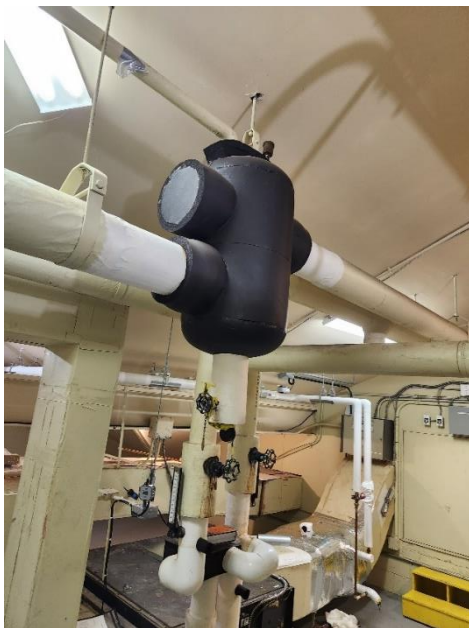
Photograph #12 – Chilled Water System Air Separator
