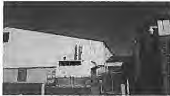
Photograph #2 – Existing RTU #2
