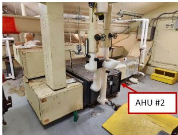
Photograph #19 – Air Handling Unit #2
