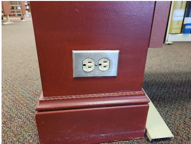
Photograph #38 - Typical Receptacle in Stacks Area
