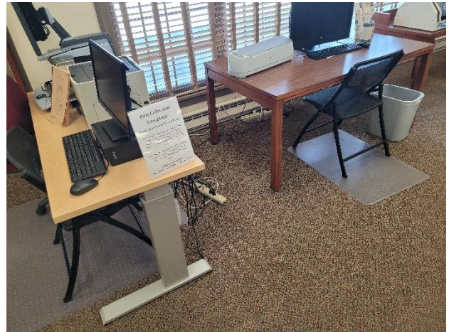
Photograph #39 - Typical Power Strips to serve computers
