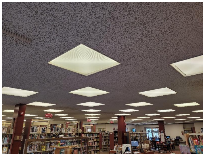
Photograph #41 - 2'x2' Lighting Fixtures
