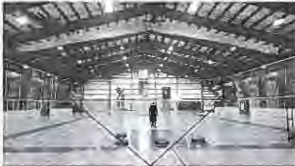
Photograph #4 – Non-Metallic Duct System with Blue DuctSox
