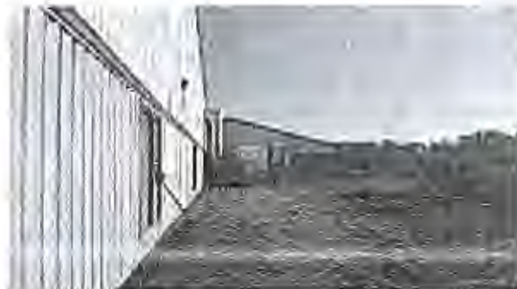
Photograph #7 – Smoke Evacuation Intake Louver
