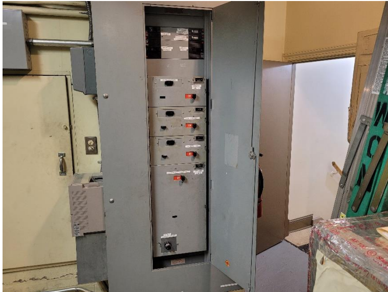
Photograph #36 – Motor Control Center MSP
