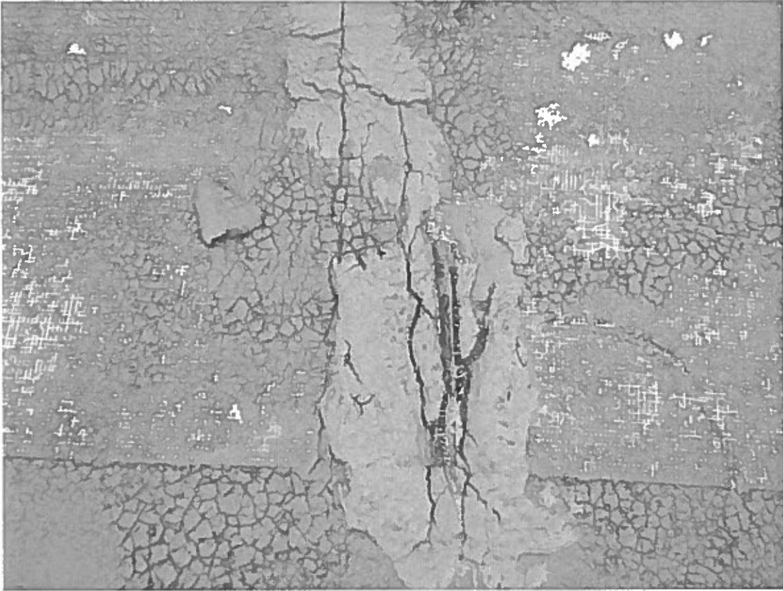
Photo 1 - Built up roof poor condition
