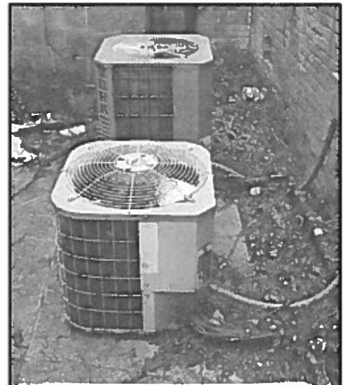
Photograph #6: Existing Condensing Units
