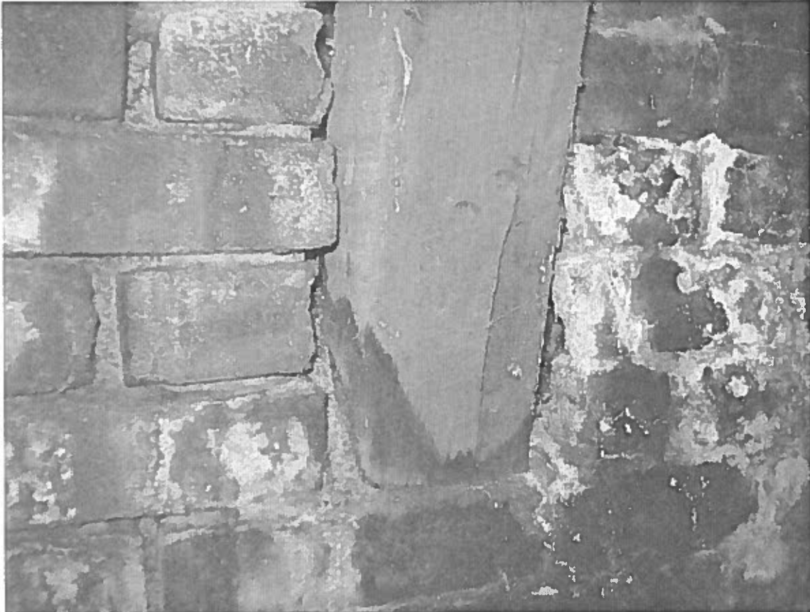
Photo 36 - Timber joist ends deteriorated
