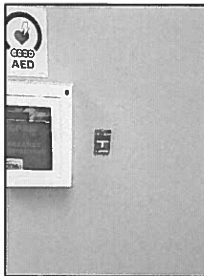
Photograph #19: Initiating Device – Manual Pull Station
