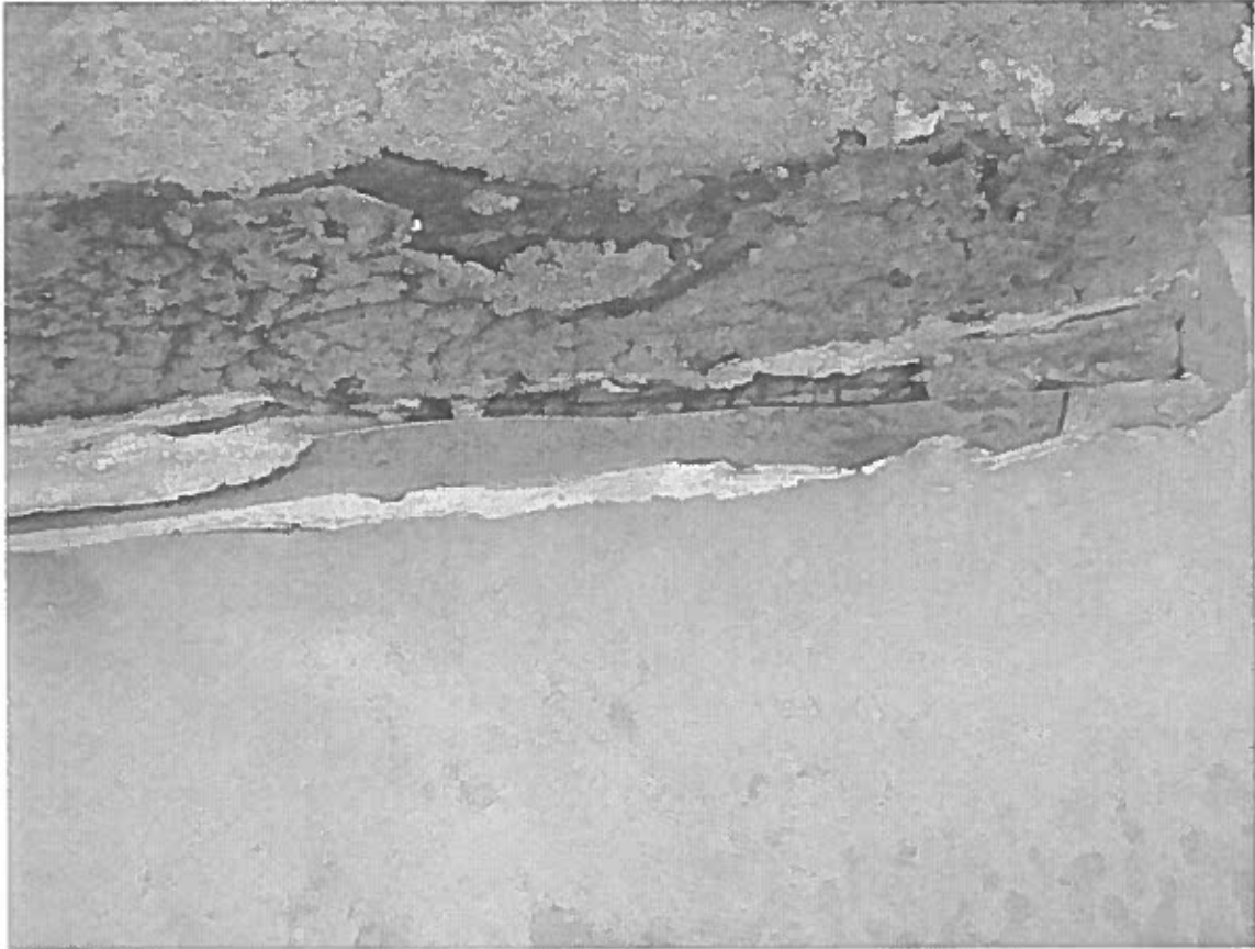
Photo 6 - Parapet wall coping open joints
