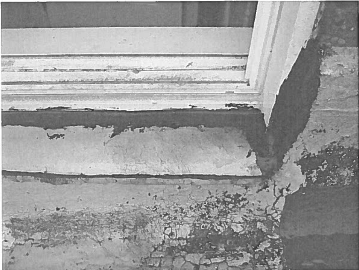
Photo 58 - Areas of water infiltration
