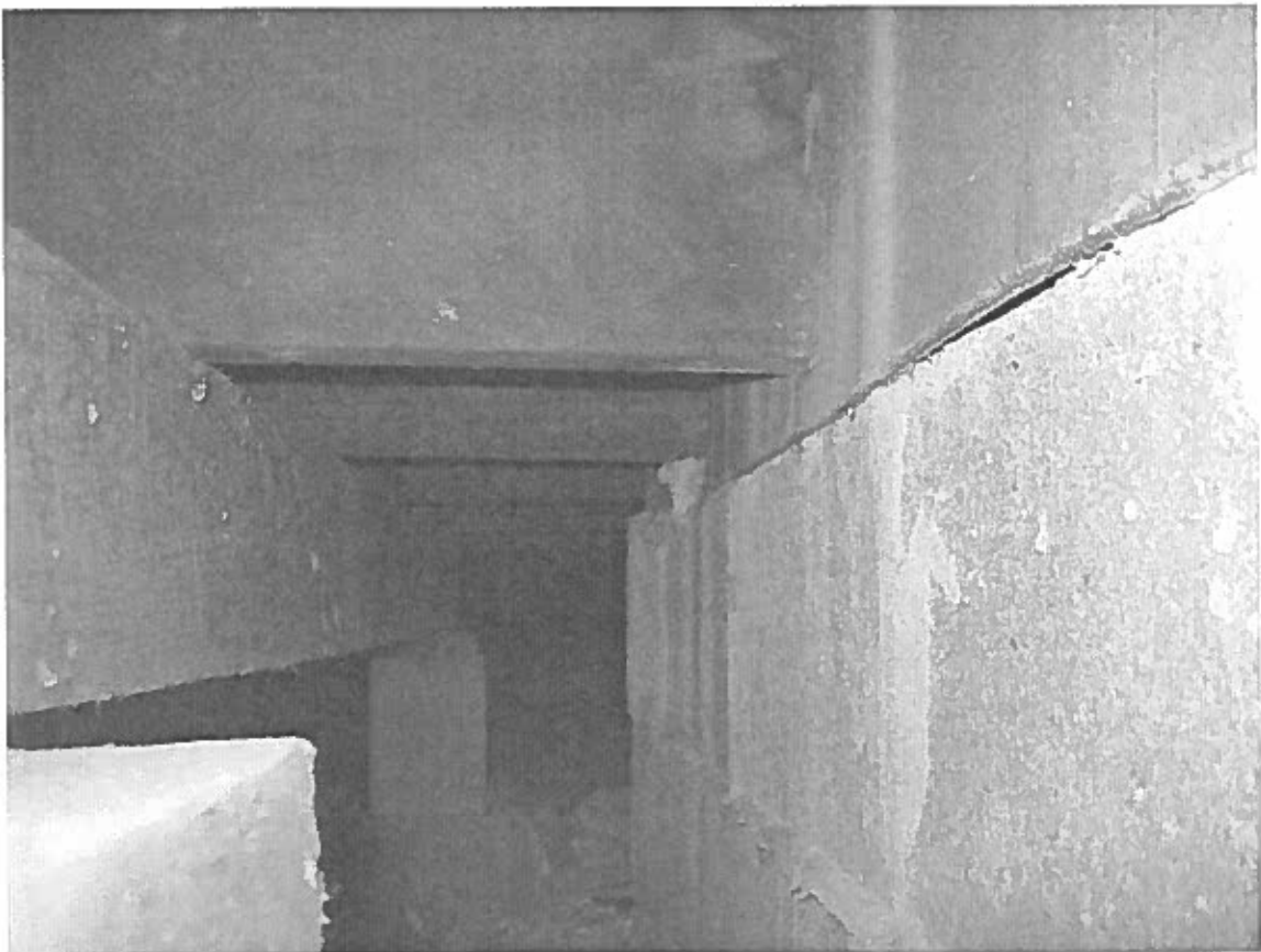
Photo 34 - Joist cut and improperly supported
