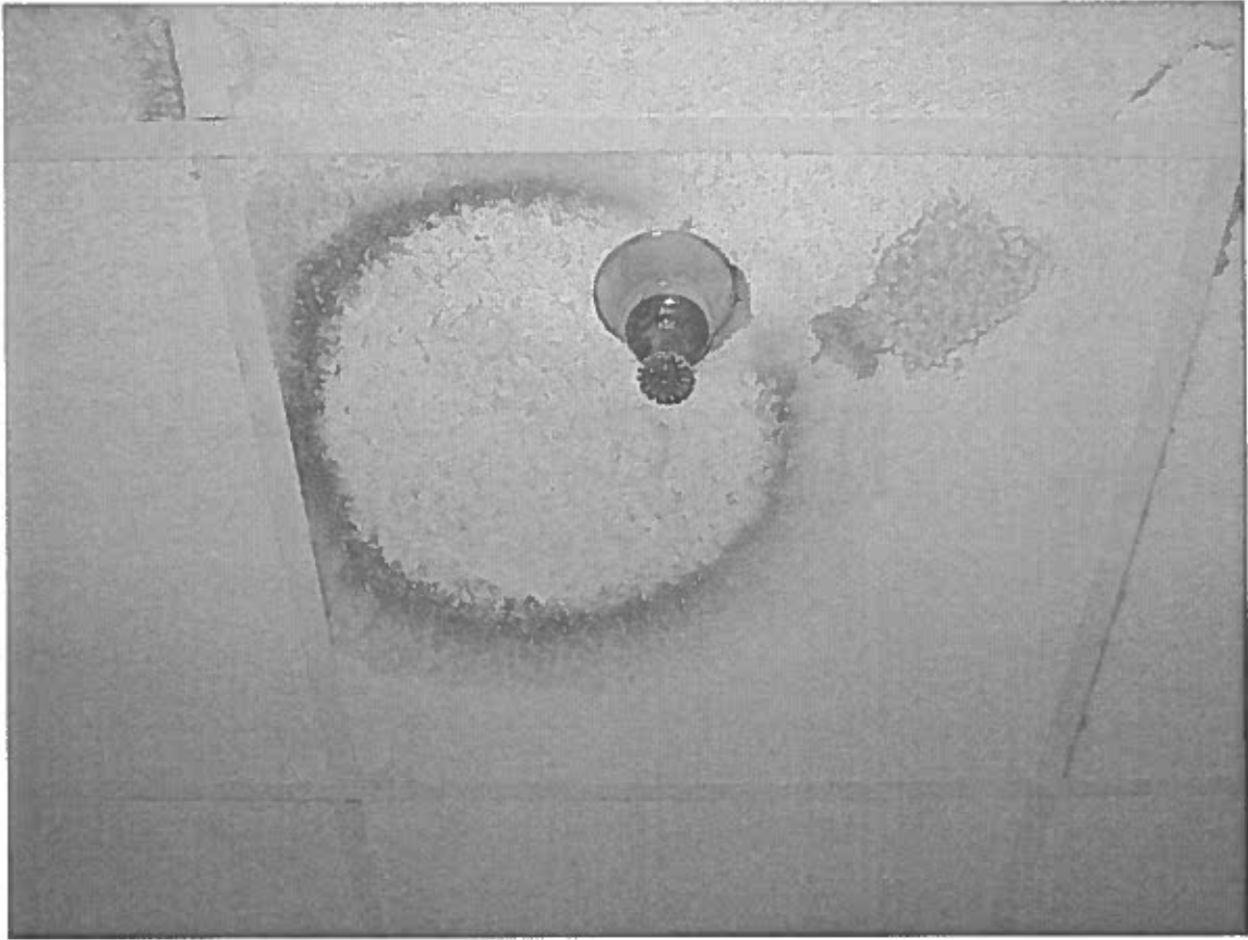
Photo 17 - Numerous water stains above third floor
