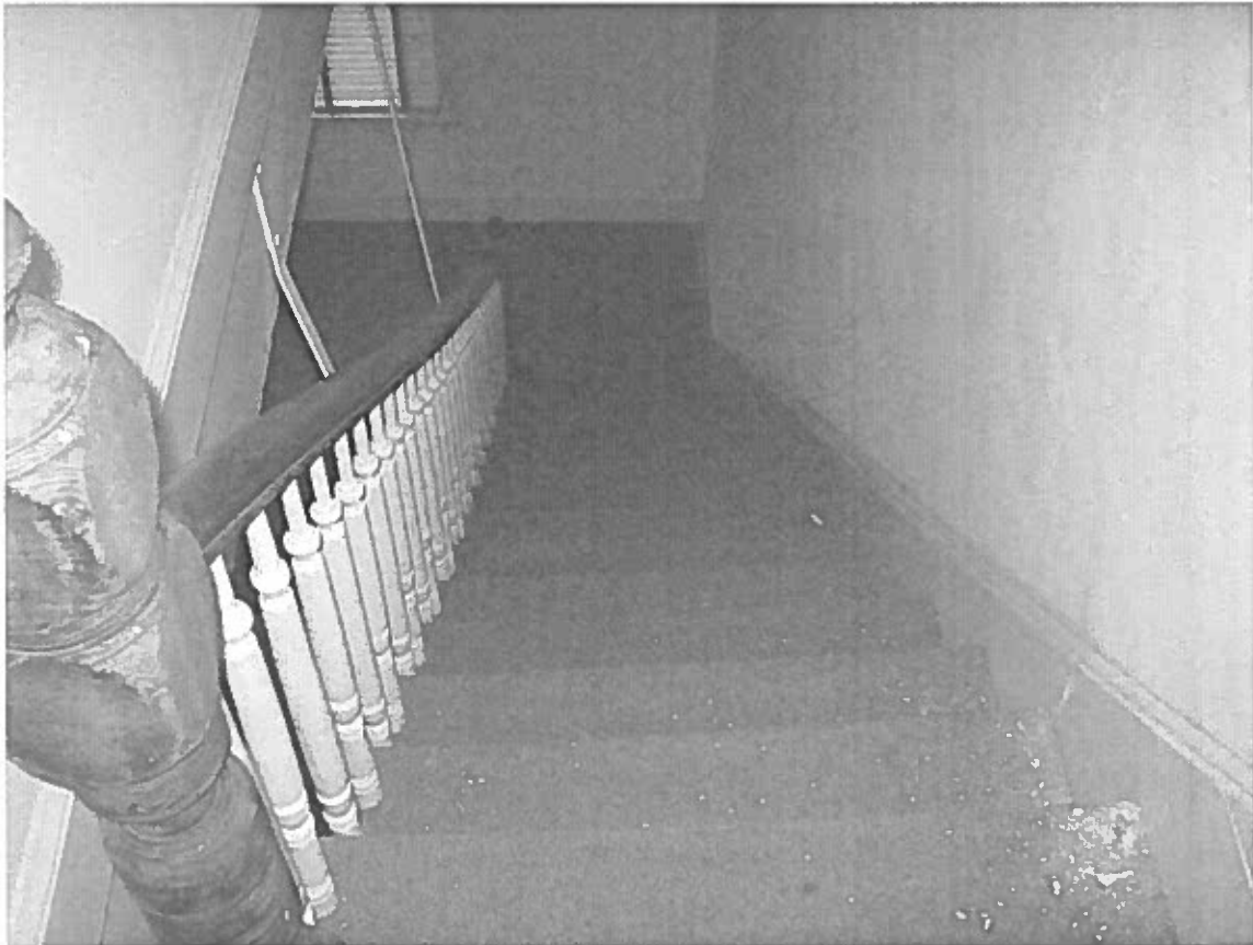
Photo 50 - Supplemental hangers for stair out of level
