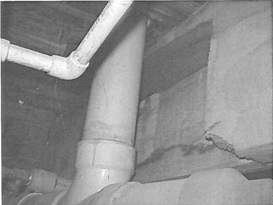
Photo 42 - Joists cut for plumbing
