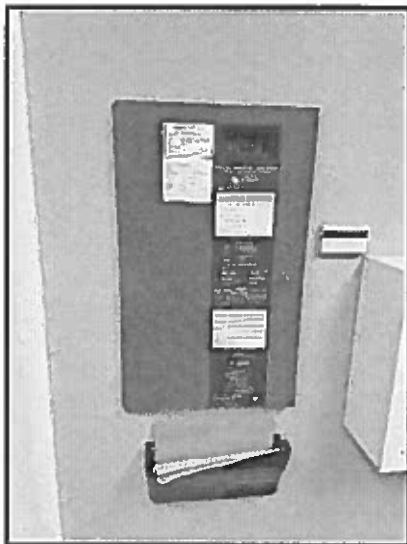
Photograph #18: Silent Knight Fire Alarm Control Panel
