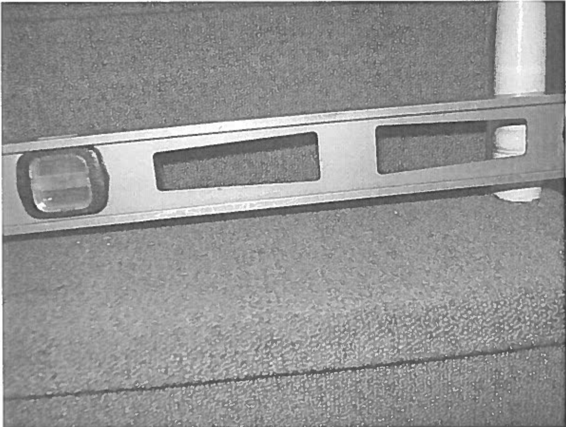
Photo 52 - Supplemental hangers for stair out of level
