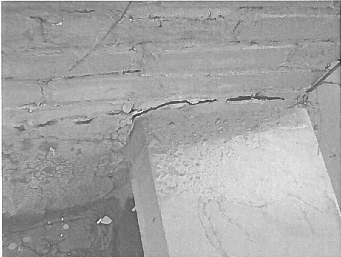
Photo 8 - Flashing and coping ends in poor condition
