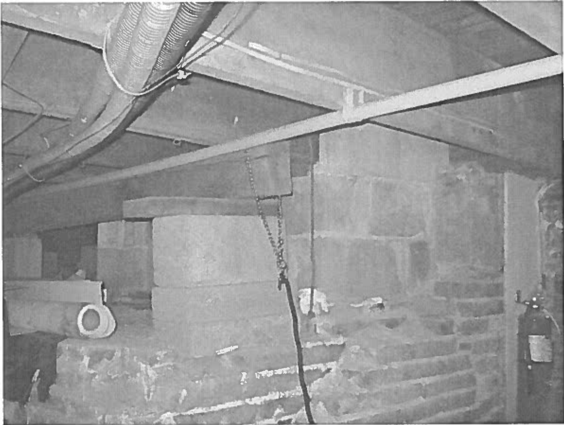
Photo 33 - Joist cut and improperly supported
