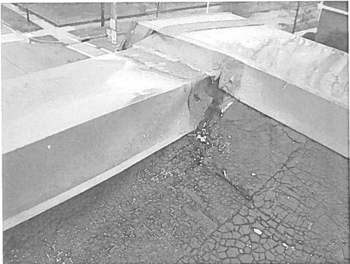
Photo 4 - Parapet wall coping open joints
