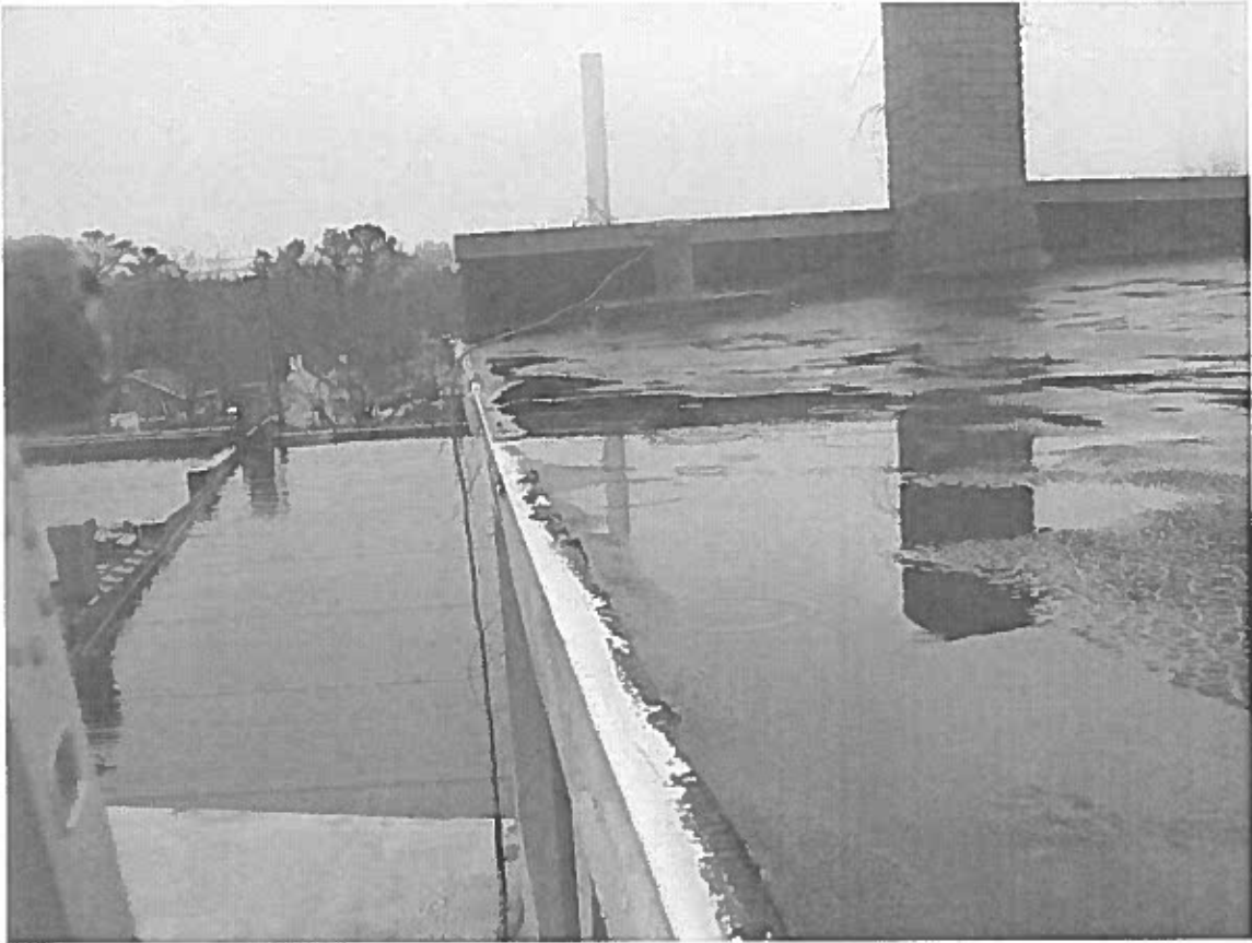
Photo 11 - Water ponding at drip edge
