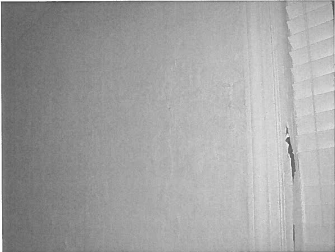
Photo 62 - Water and moisture infiltration affecting finishes
