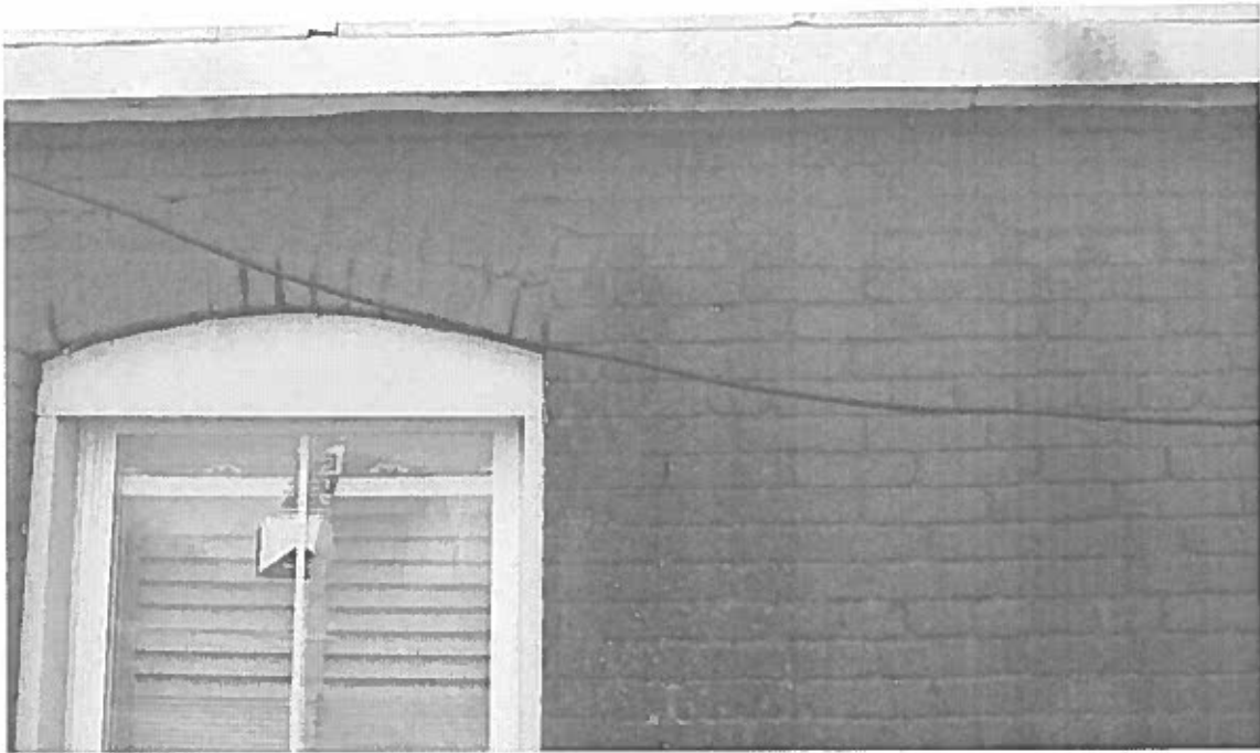
Photo 57 - Areas of water infiltration
