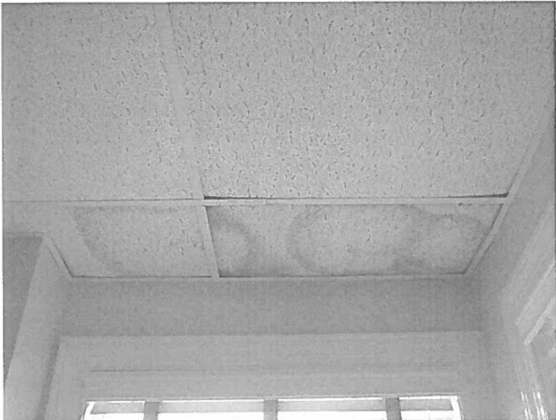
Photo 64 - Water and moisture infiltration affecting finishes
