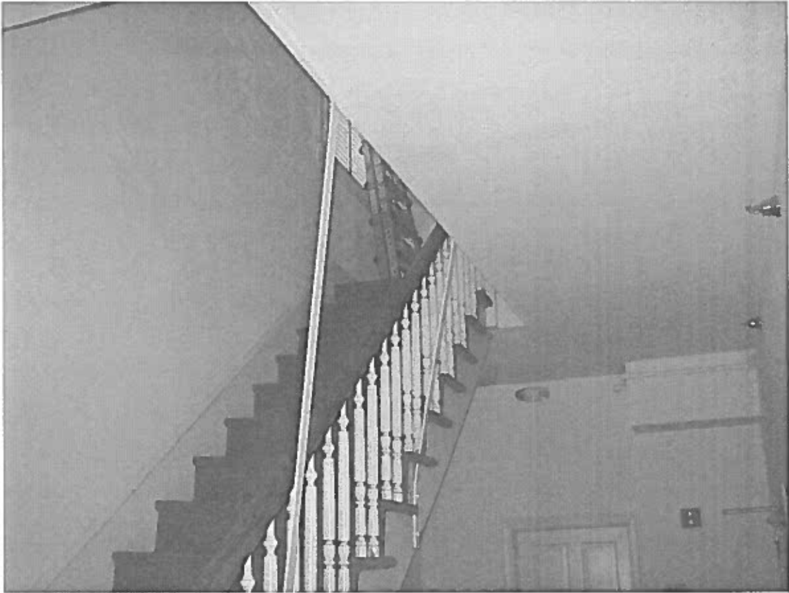
Photo 49 - Supplemental hangers for stair out of level
