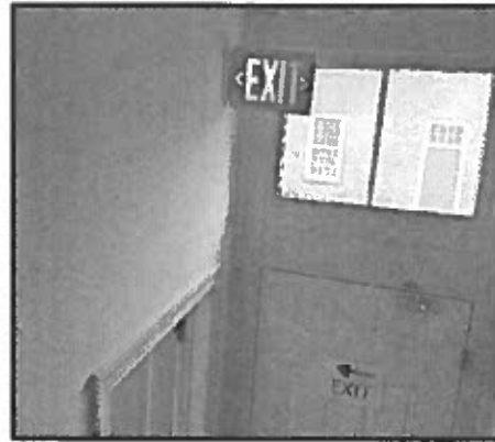
Photograph #17: Exit Sign with Integral Battery Backup
