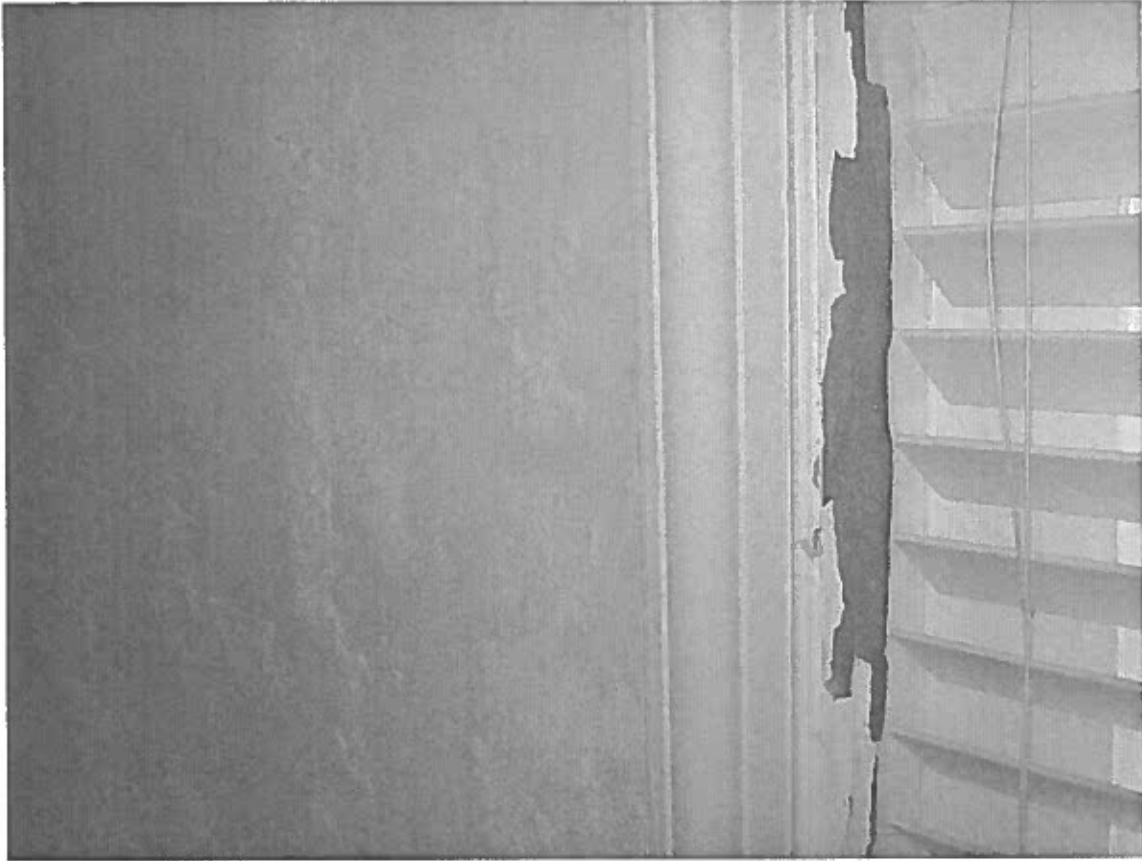
Photo 63 - Water and moisture infiltration affecting finishes
