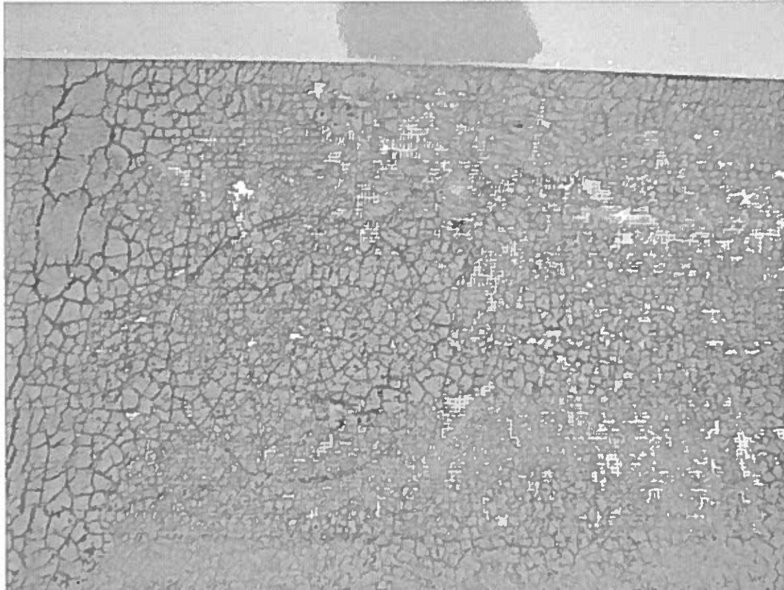
Photo 2 - Built up roof poor condition
