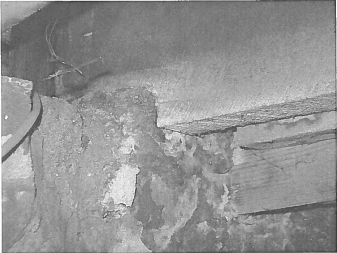
Photo 39 - Joist end deterioration due to moisture
