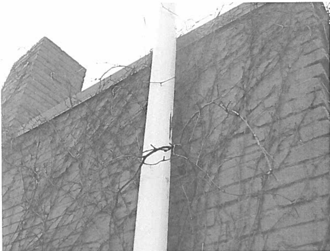
Photo 60 - Vines at building corner and loose vent stack
