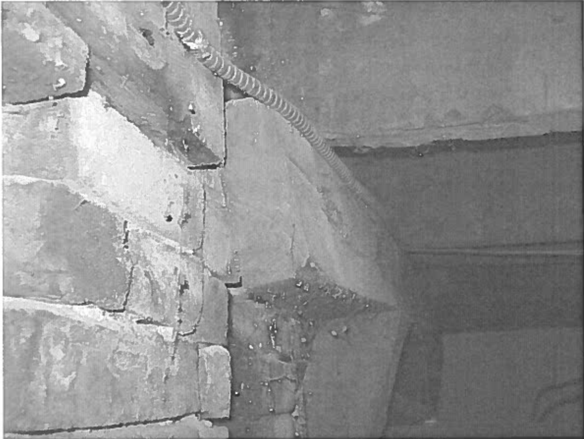
Photo 37 - Timber joist ends deteriorated
