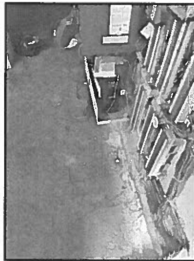
Photograph #23: Uninterrupted Power Supply
