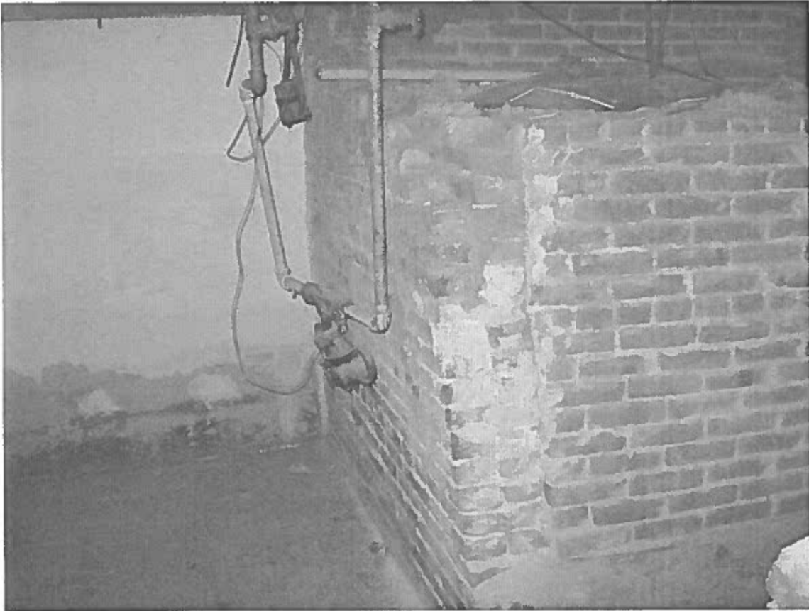
Photo 43 - Basement retaining wall leaning
