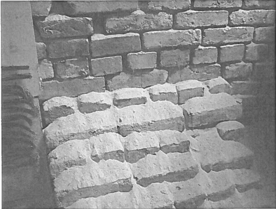
Photo 44 - Mortar joints in basement eroded
