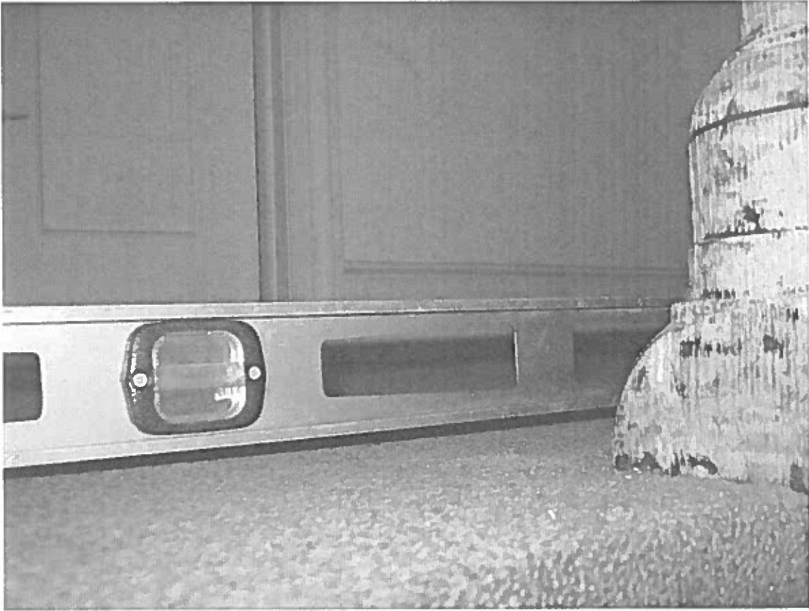
Photo 51 - Supplemental hangers for stair out of level
