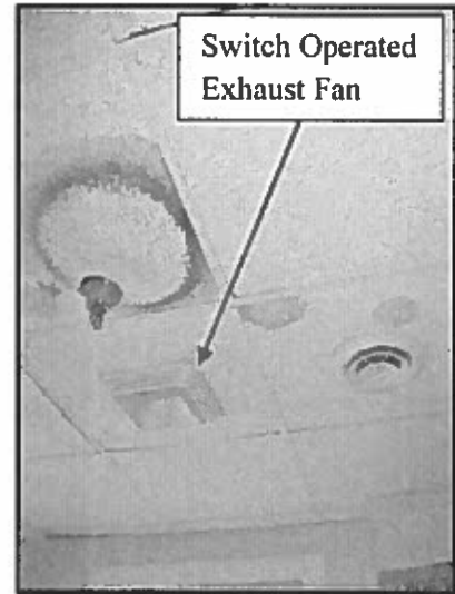
Photograph #7: Bathroom Exhaust Fan
