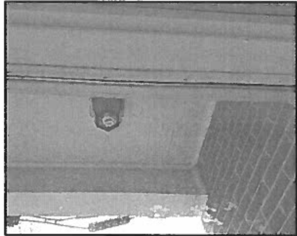
Photograph #14: Exterior Light
