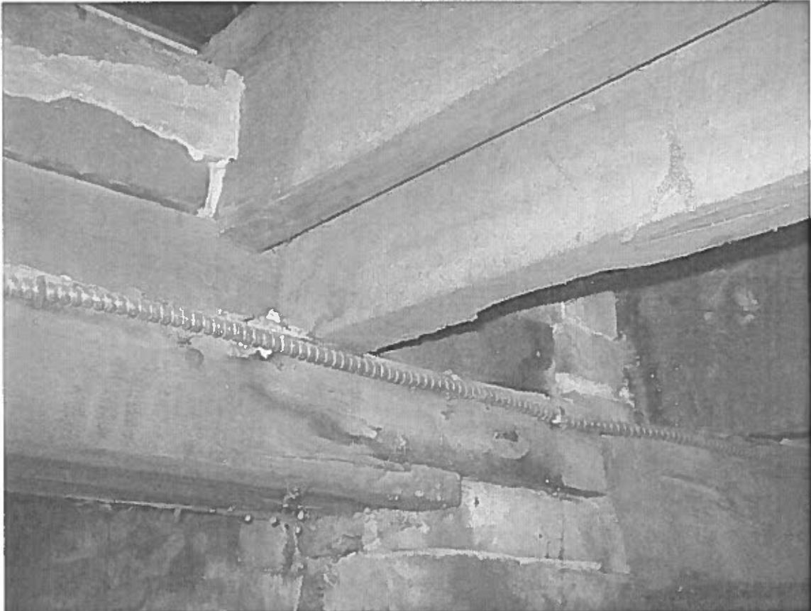
Photo 38 - Timber joist ends deteriorated
