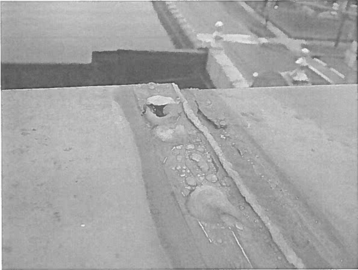
Photo 5 - Parapet wall coping open joints
