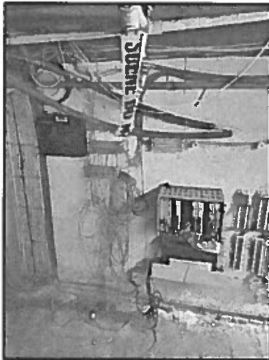
Photograph #22: Fiber Cabling and Network Gear
