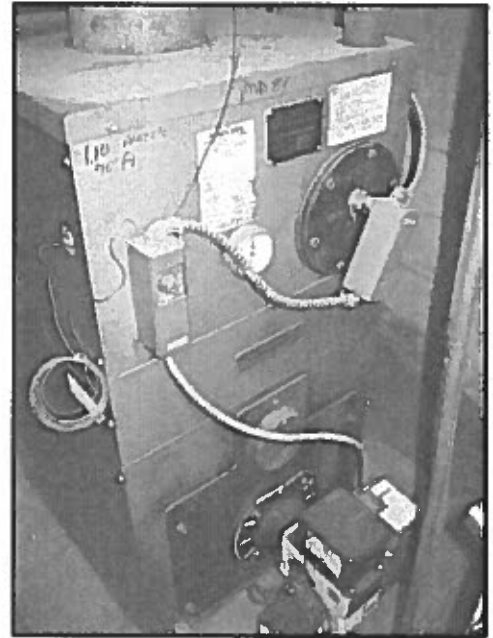
Photograph #2: Existing Fuel Oil Fired Boiler
