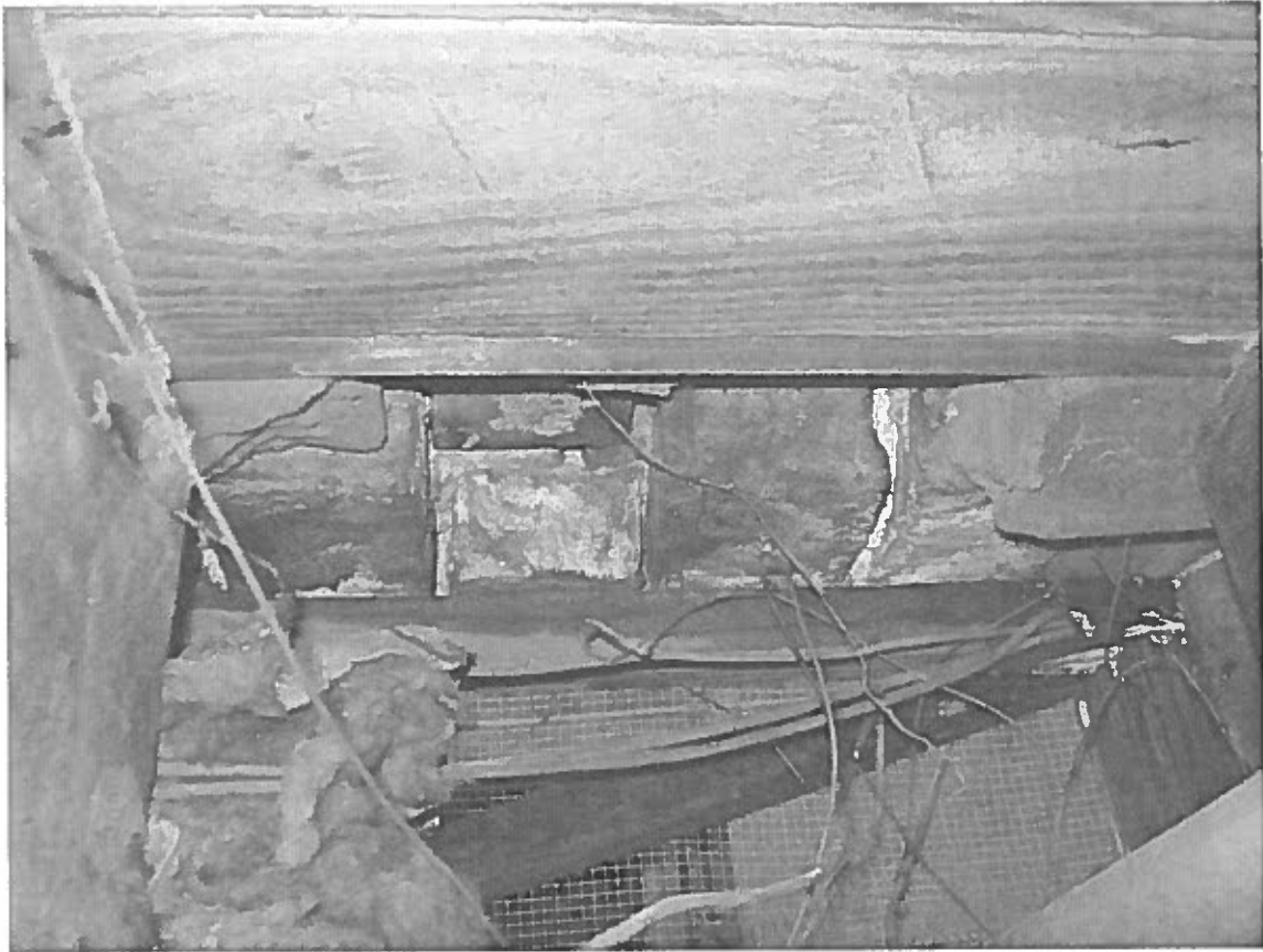
Photo 41 - Openings in mechanical room allowing water infiltration
