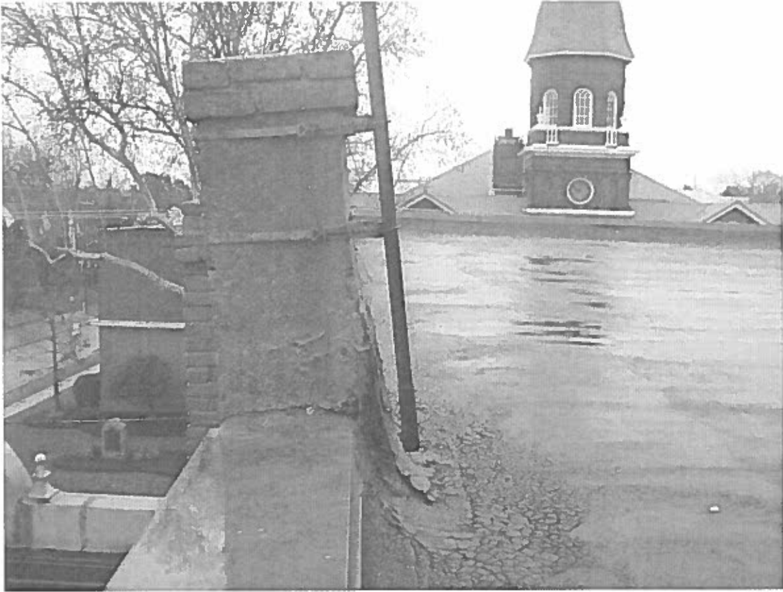
Photo 9 - Leaning brick chimney
