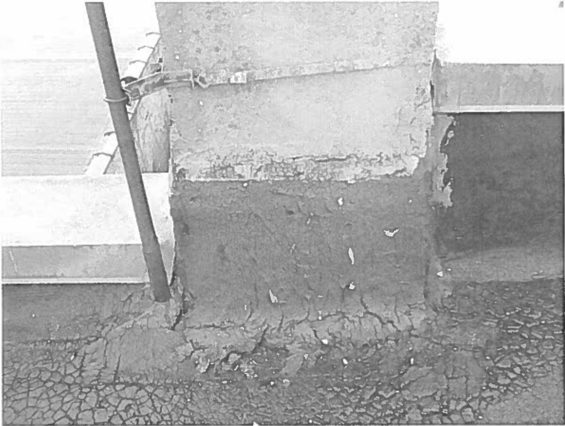
Photo 7 - Flashing and coping ends in poor condition
