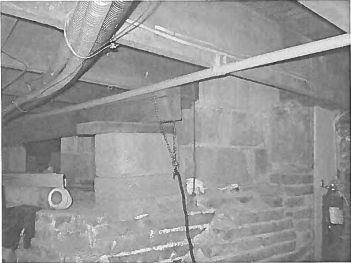
Photo 33 - Joist cut and improperly supported
