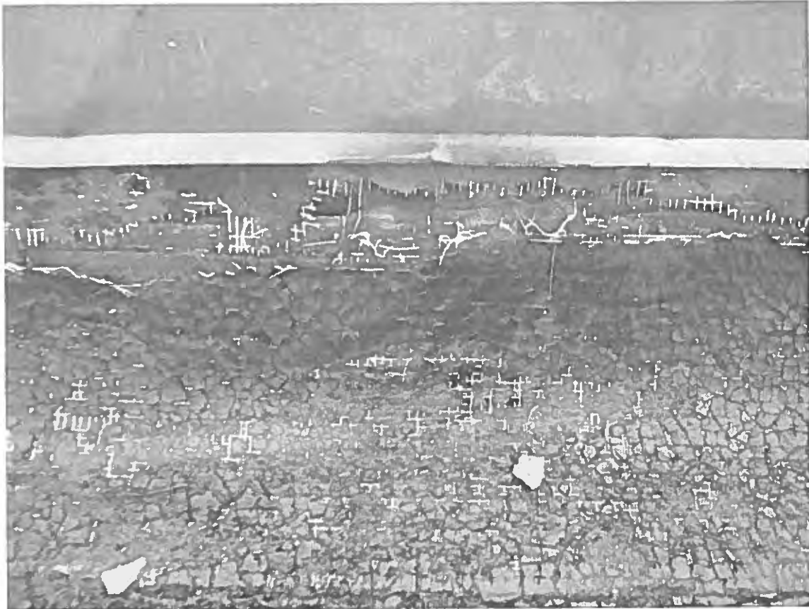
Photo 3 - Built up roof poor condition
