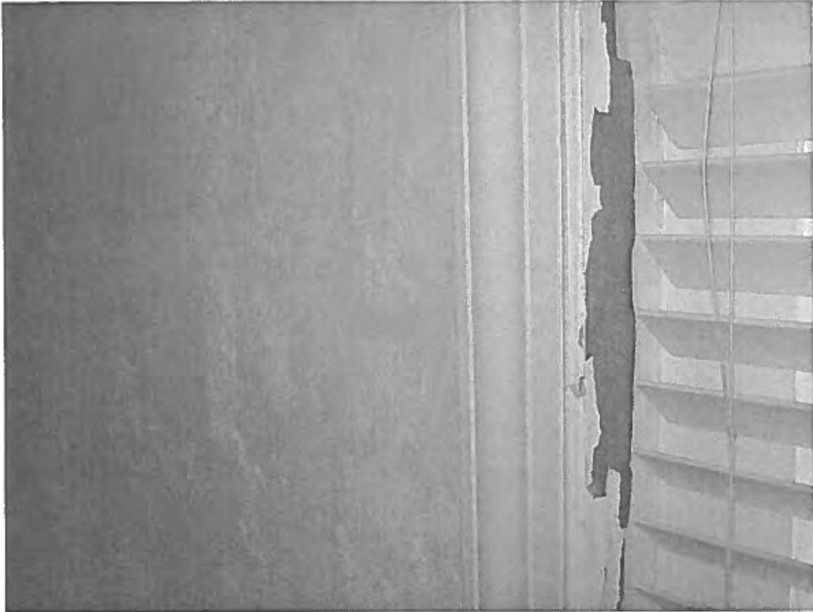
Photo 63 - Water and moisture infiltration affecting finishes
