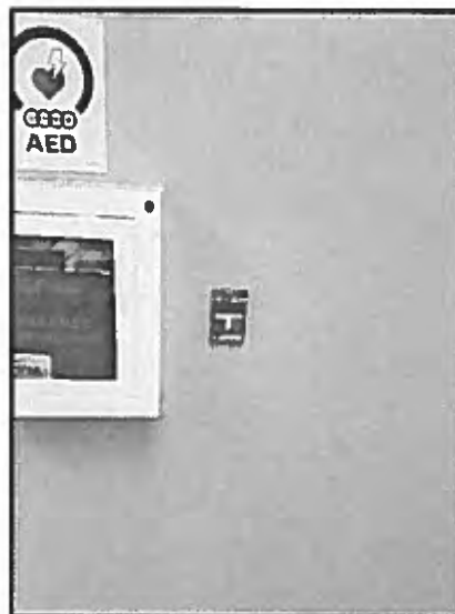
Photograph #19: Initiating Device – Manual Pull Station
