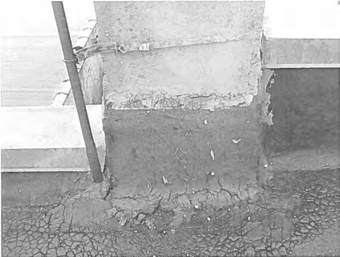
Photo 7 - Flashing and coping ends in poor condition
