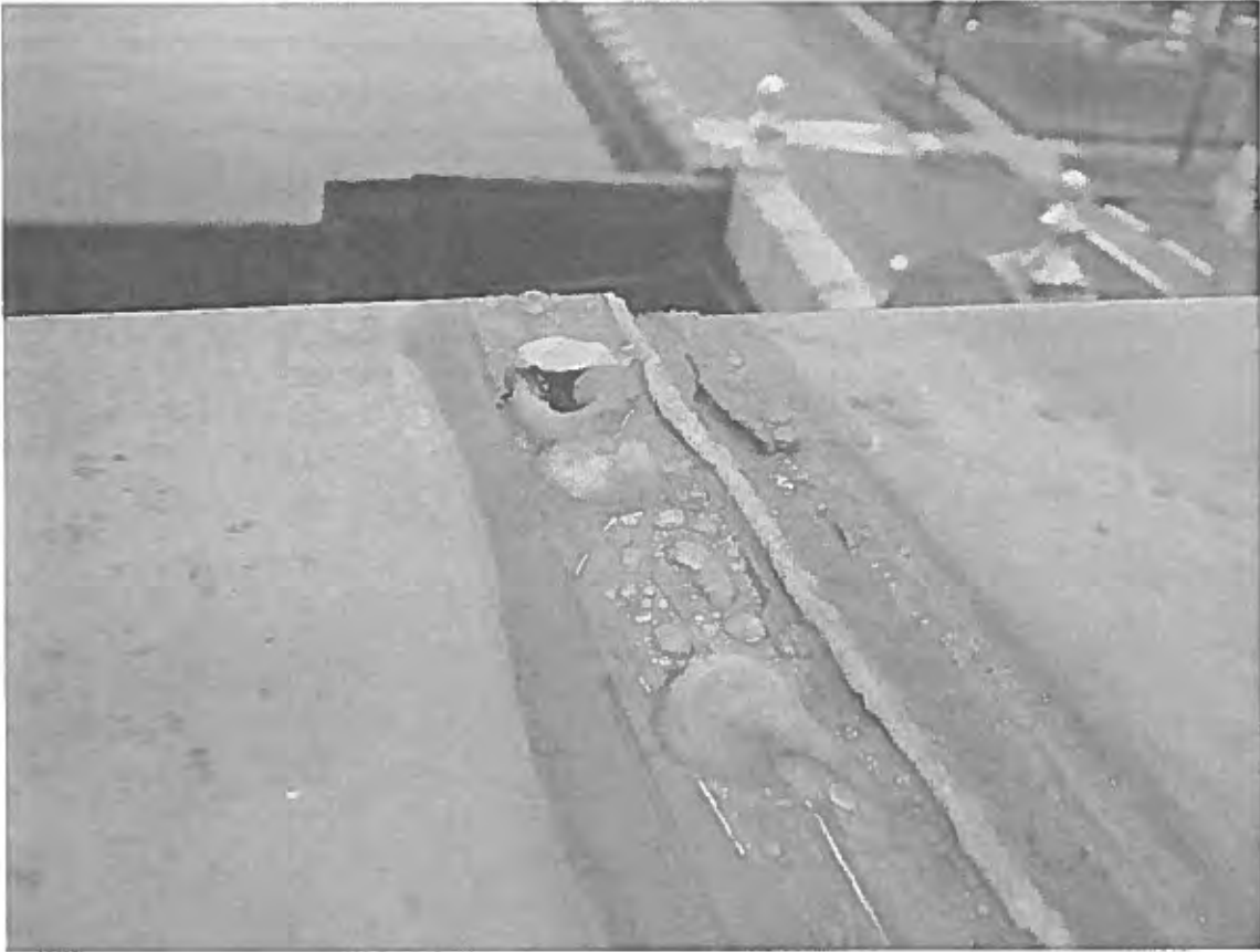
Photo 5 - Parapet wall coping open joints
