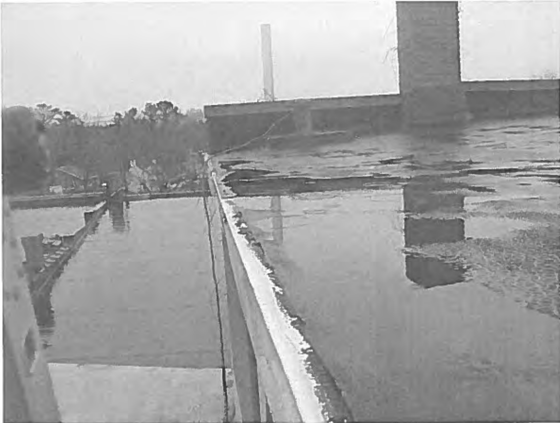
Photo 11 - Water ponding at drip edge
