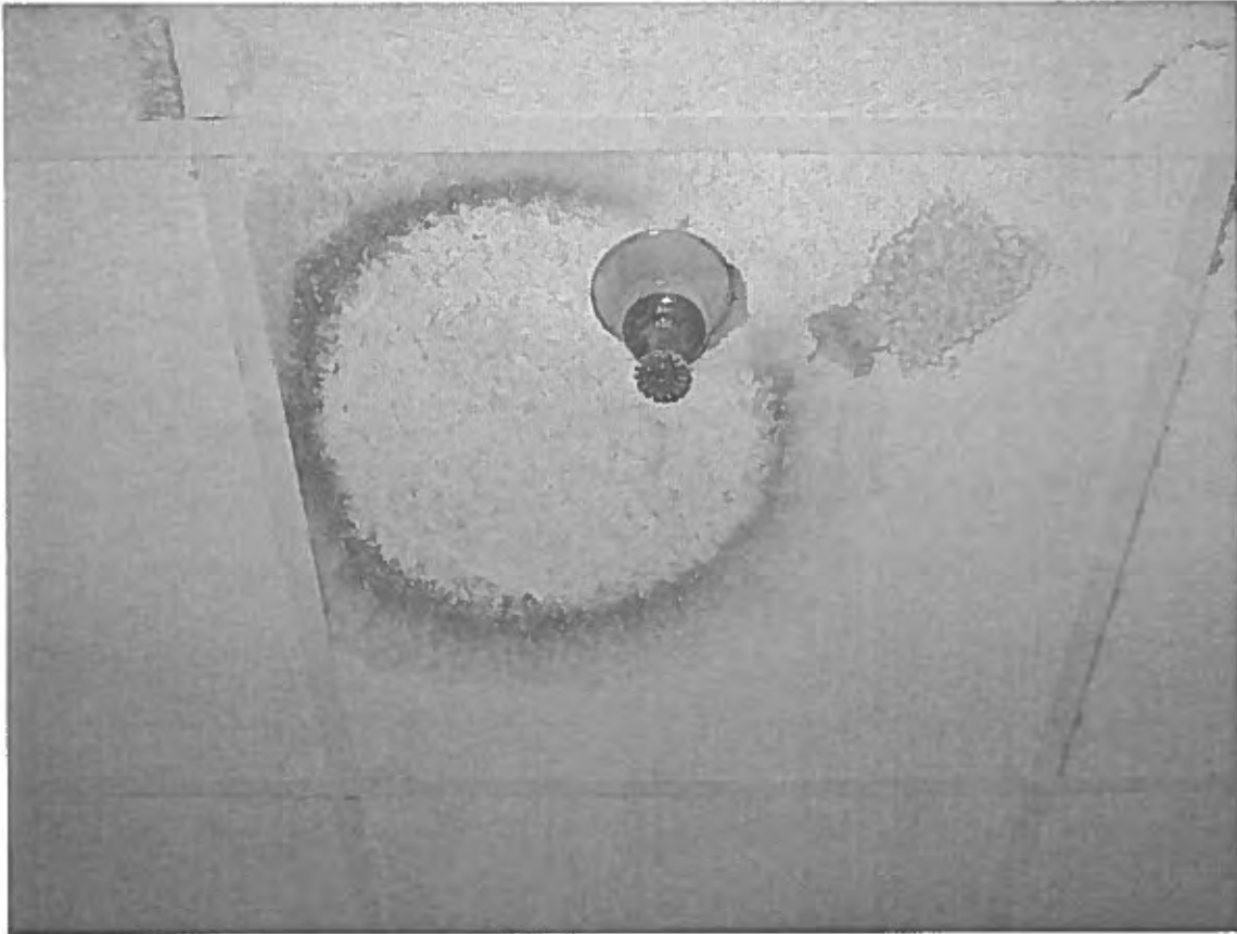
Photo 17 - Numerous water stains above third floor
