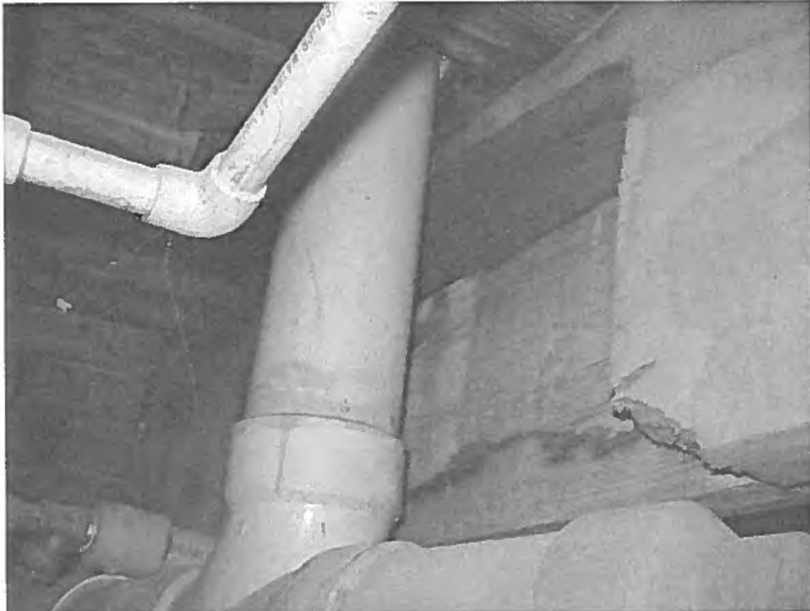
Photo 42 - Joists cut for plumbing
