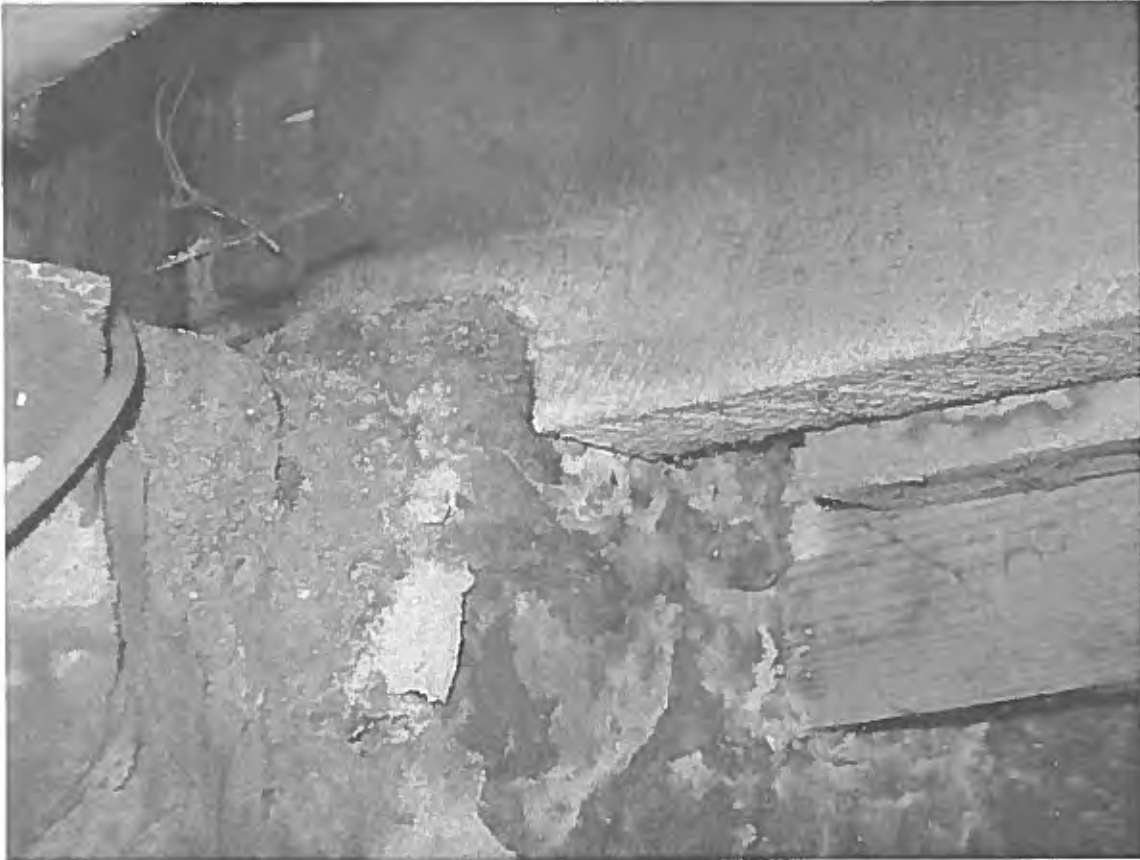
Photo 39 - Joist end deterioration due to moisture
