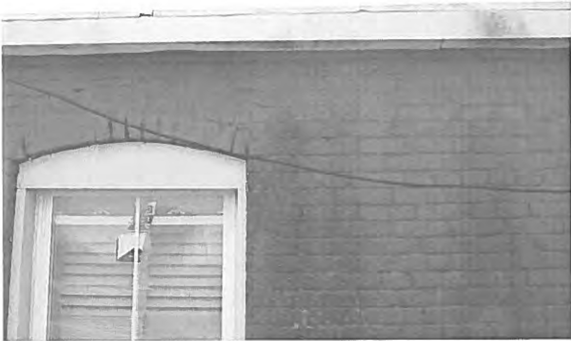
Photo 57 - Areas of water infiltration
