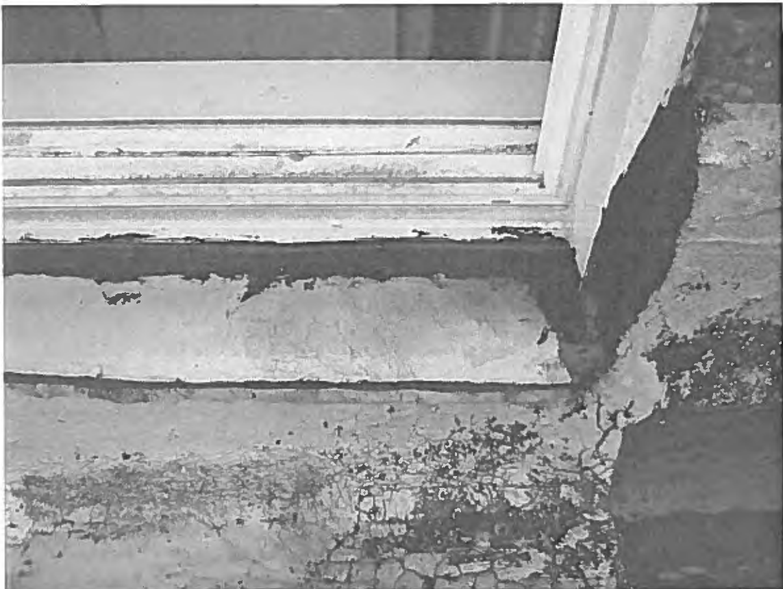
Photo 58 - Areas of water infiltration
