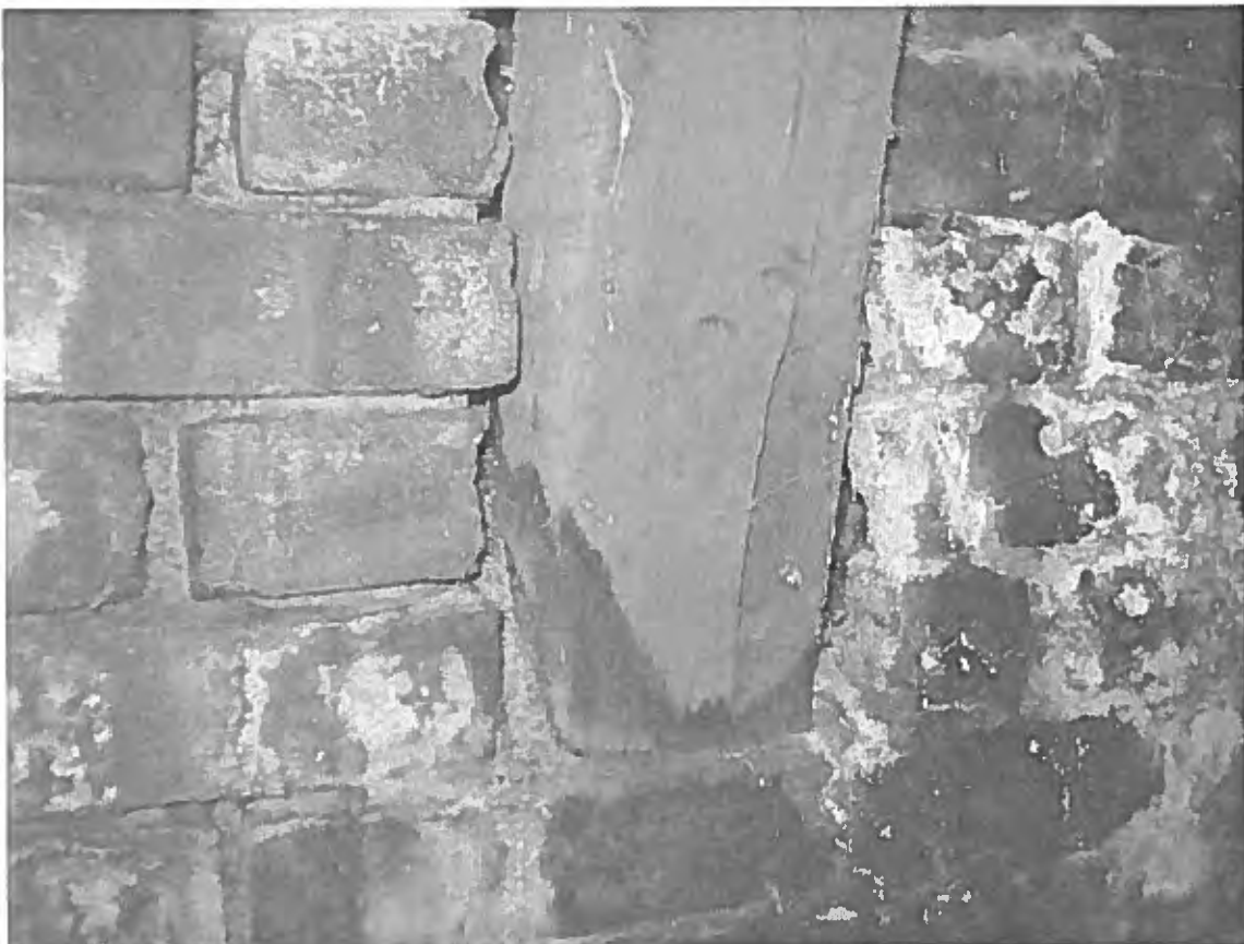
Photo 36 - Timber joist ends deteriorated
