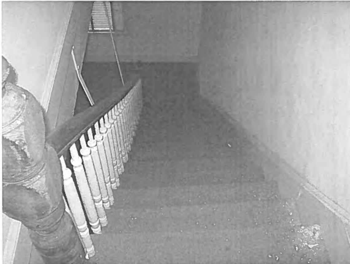
Photo 50 - Supplemental hangers for stair out of level
