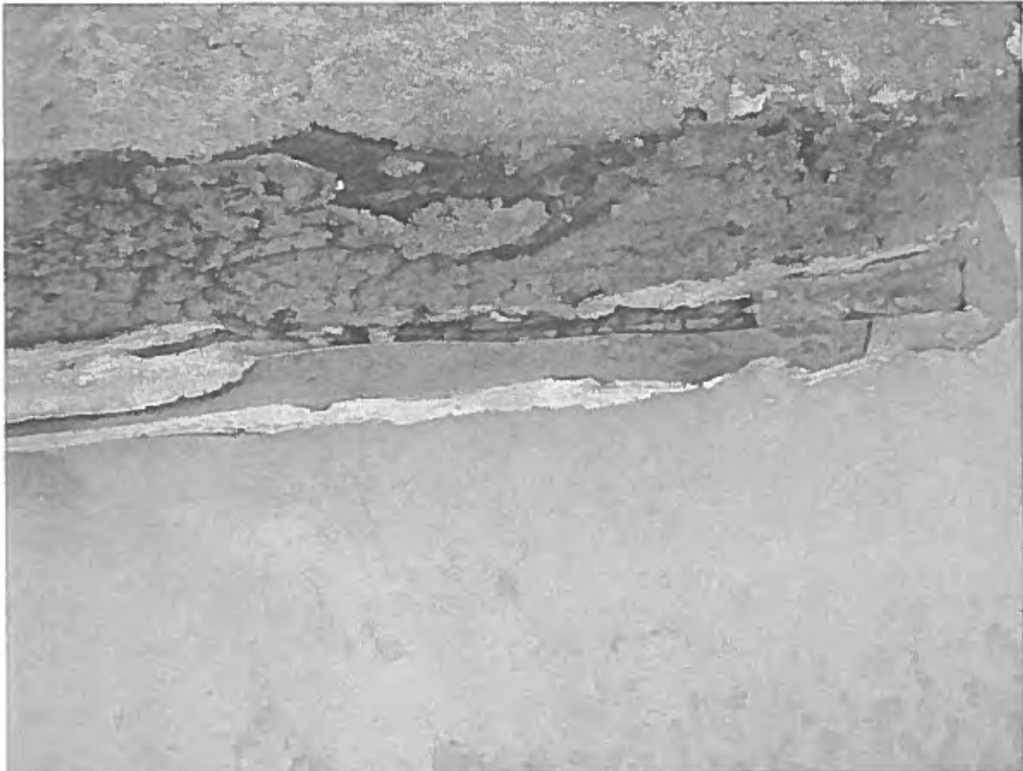
Photo 6 - Parapet wall coping open joints
