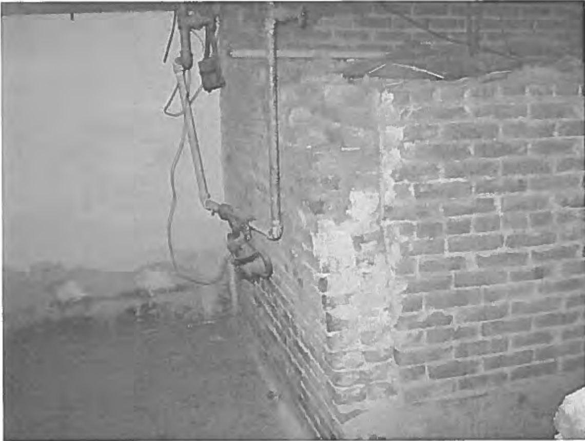
Photo 43 - Basement retaining wall leaning
