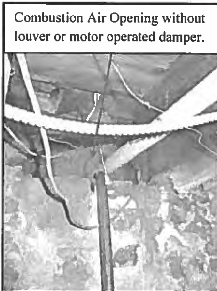
Photograph #3: Un-protected Combustion Air Opening
