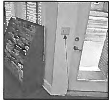
Photograph #15: Lighting Switch
