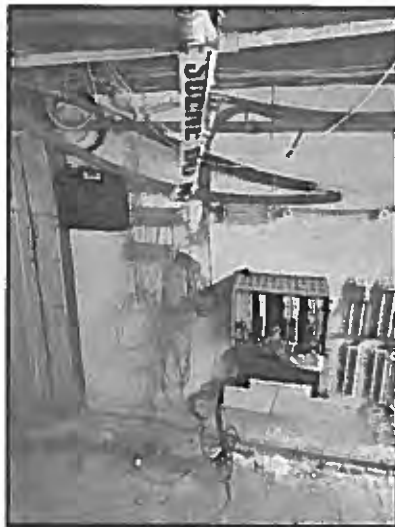
Photograph #22: Fiber Cabling and Network Gear
