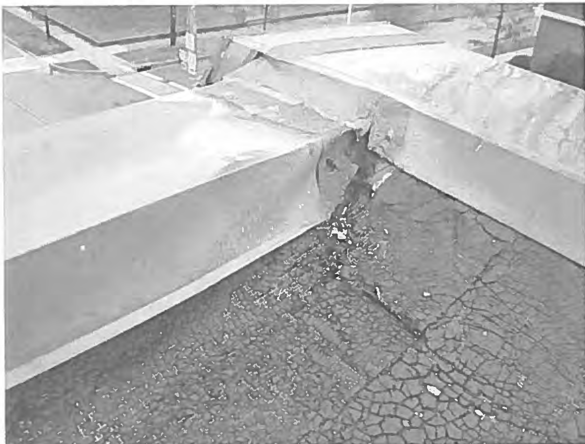
Photo 4 - Parapet wall coping open joints
