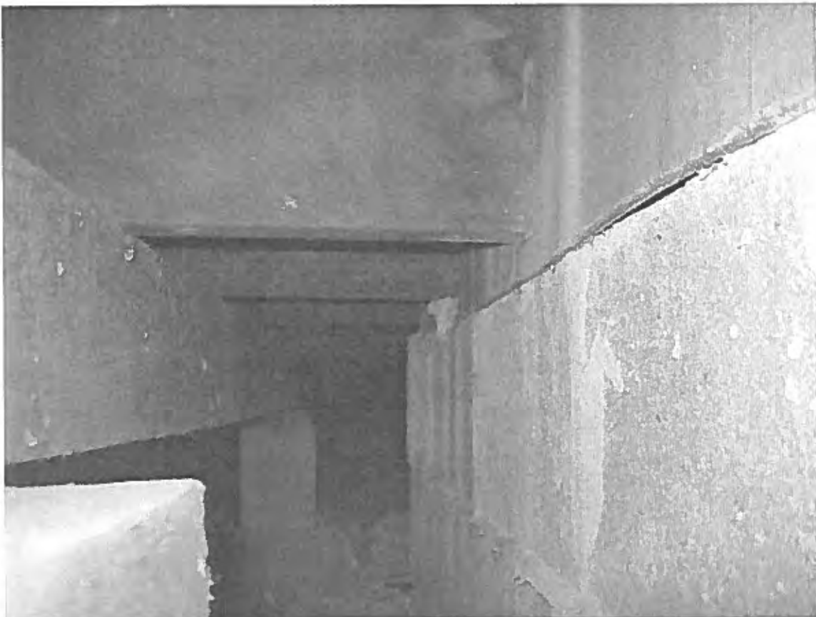
Photo 34 - Joist cut and improperly supported
