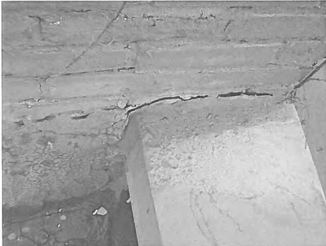
Photo 8 - Flashing and coping ends in poor condition
