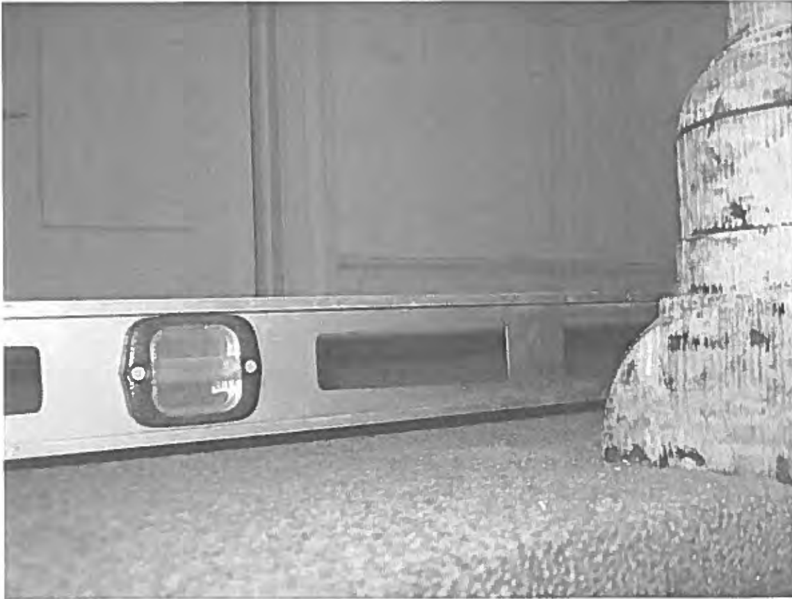
Photo 51 - Supplemental hangers for stair out of level
