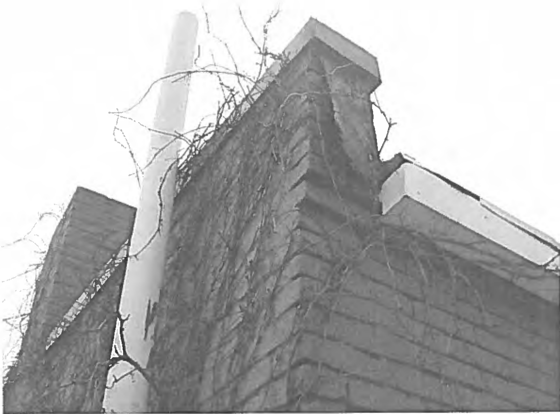
Photo 59 - Vines at building corner and loose vent stack
