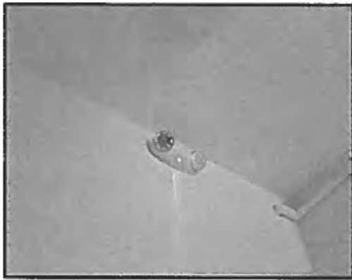
Photograph #16: Emergency Egress Lighting
