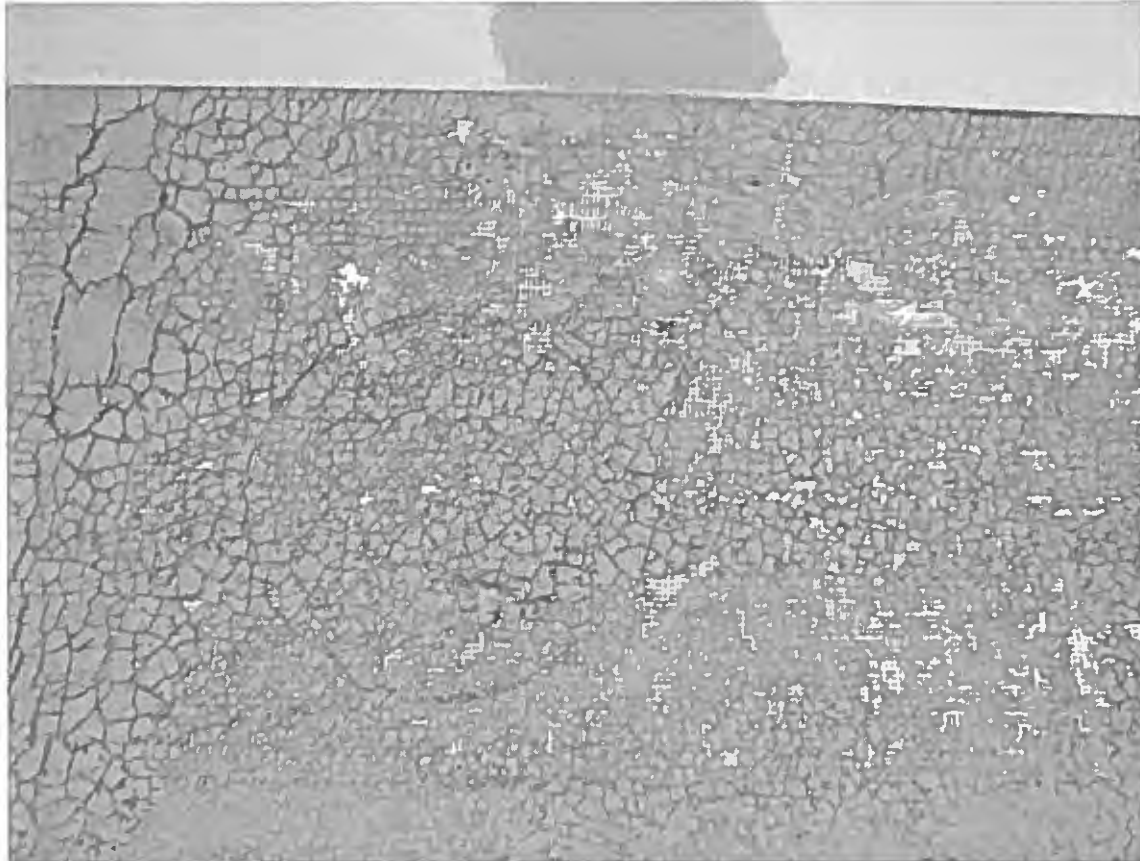
Photo 2 - Built up roof poor condition
