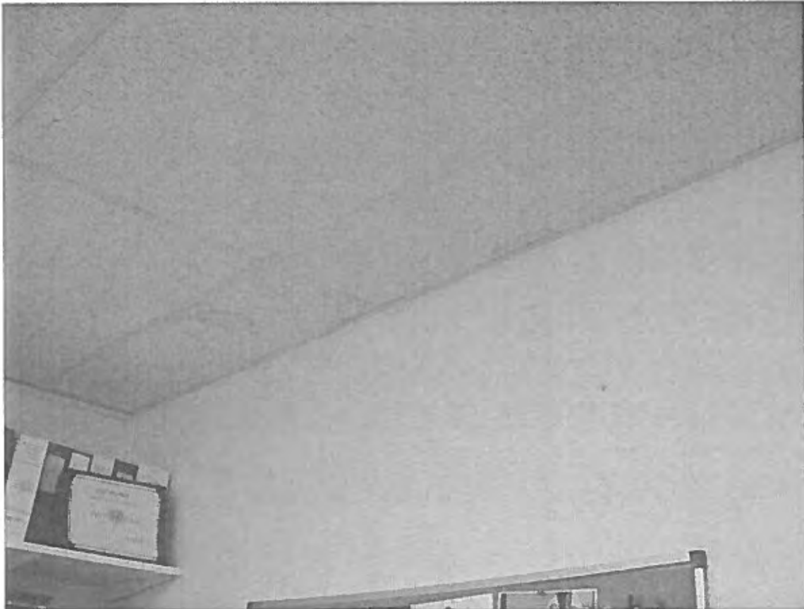
Photo 18 - Numerous water stains above third floor
