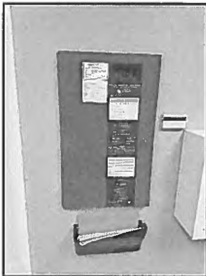
Photograph #18: Silent Knight Fire Alarm Control Panel
