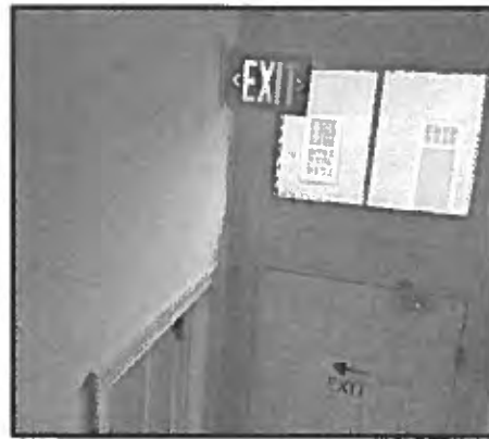
Photograph #17: Exit Sign with Integral Battery Backup
