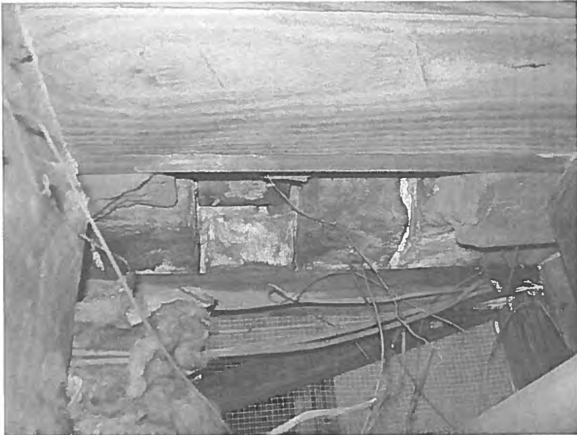
Photo 41 - Openings in mechanical room allowing water infiltration
