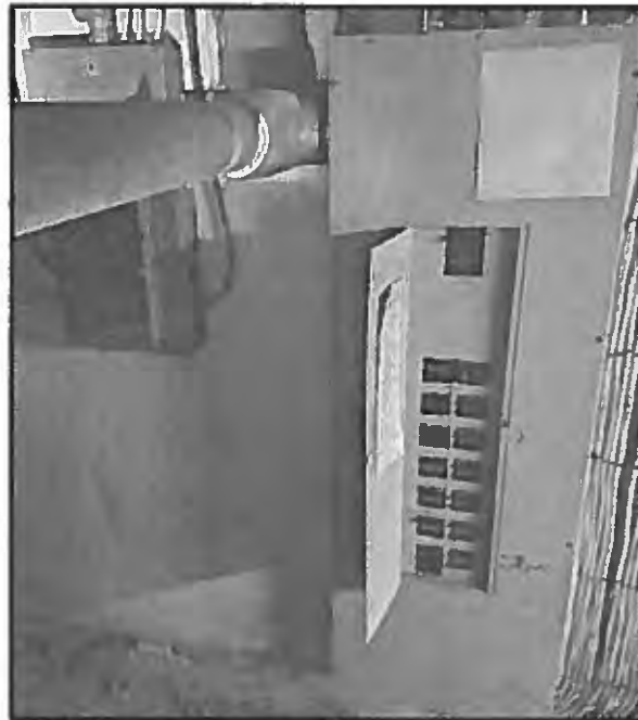
Photograph #9: General Electric 400A Panelboard
