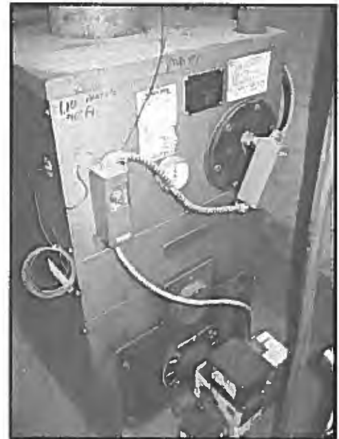
Photograph #2: Existing Fuel Oil Fired Boiler
