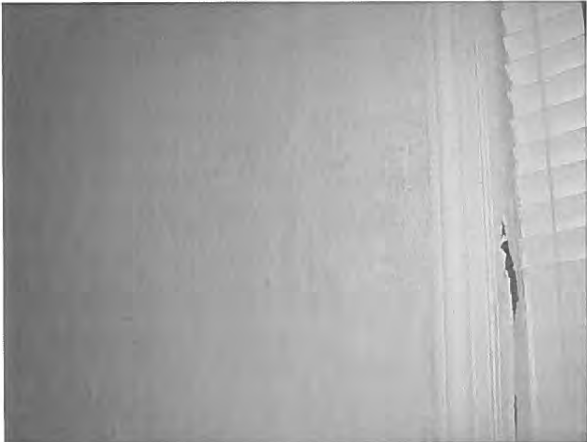
Photo 62 - Water and moisture infiltration affecting finishes
