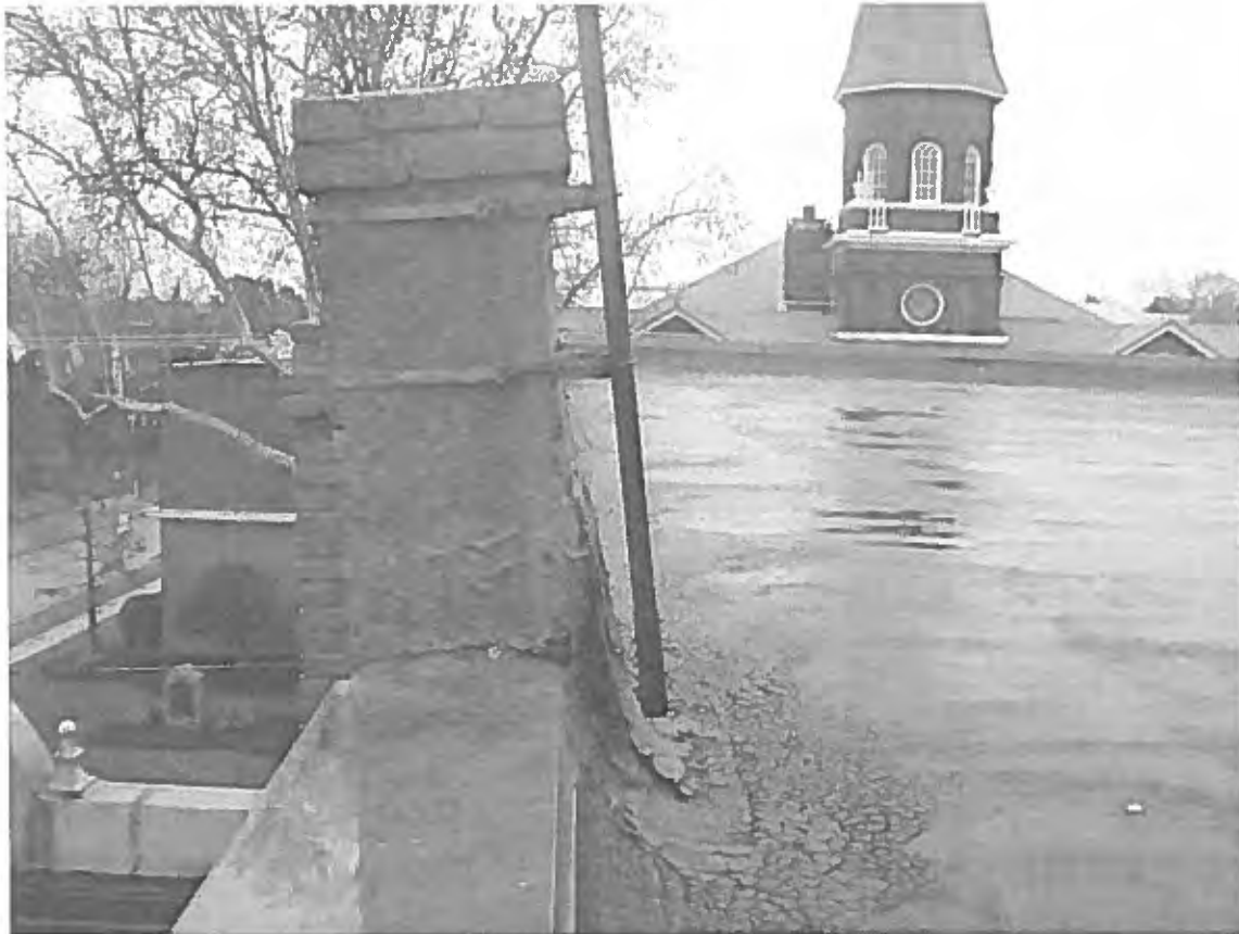
Photo 9 - Leaning brick chimney
