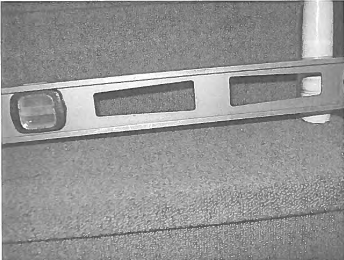
Photo 52 - Supplemental hangers for stair out of level
