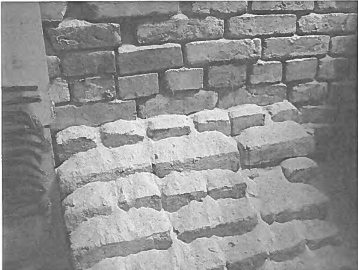
Photo 44 - Mortar joints in basement eroded
