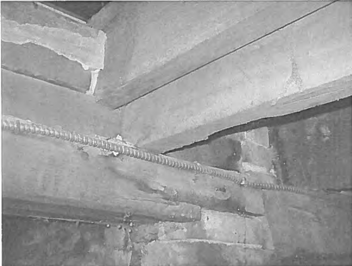
Photo 38 - Timber joist ends deteriorated
