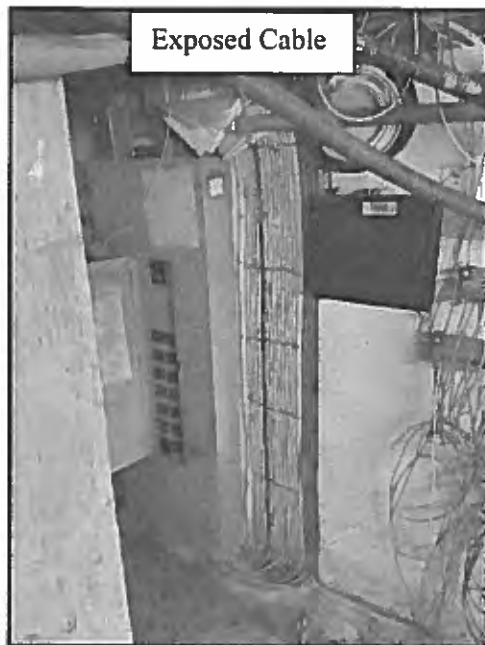
Photograph #10: Example of Non-Metallic Sheathed Cable
