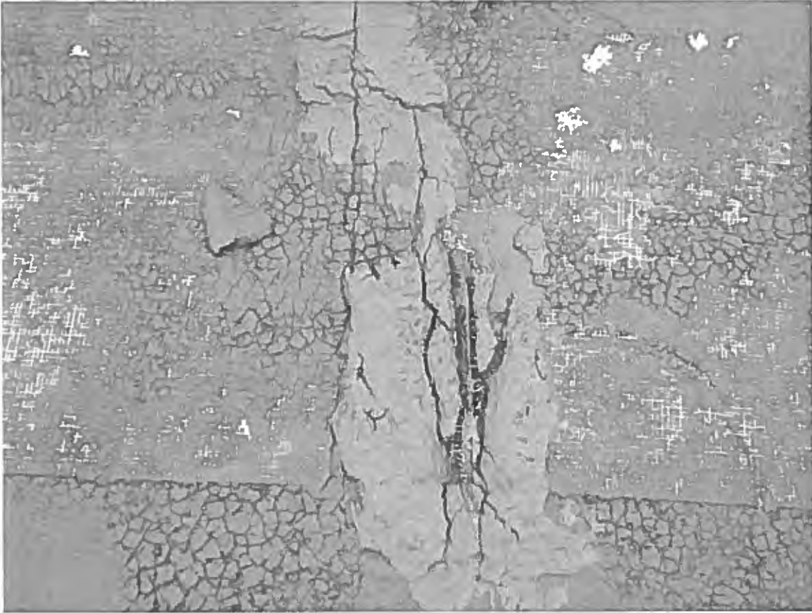
Photo 1 - Built up roof poor condition
