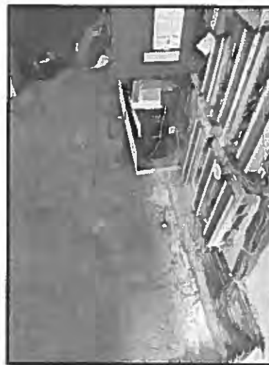
Photograph #23: Uninterrupted Power Supply
