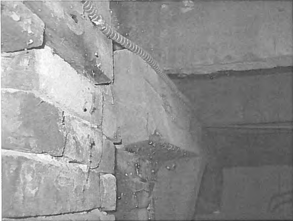
Photo 37 - Timber joist ends deteriorated
