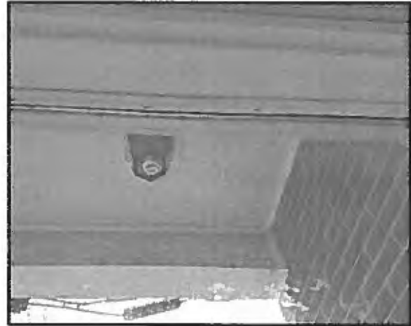
Photograph #14: Exterior Light
