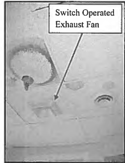
Photograph #7: Bathroom Exhaust Fan
