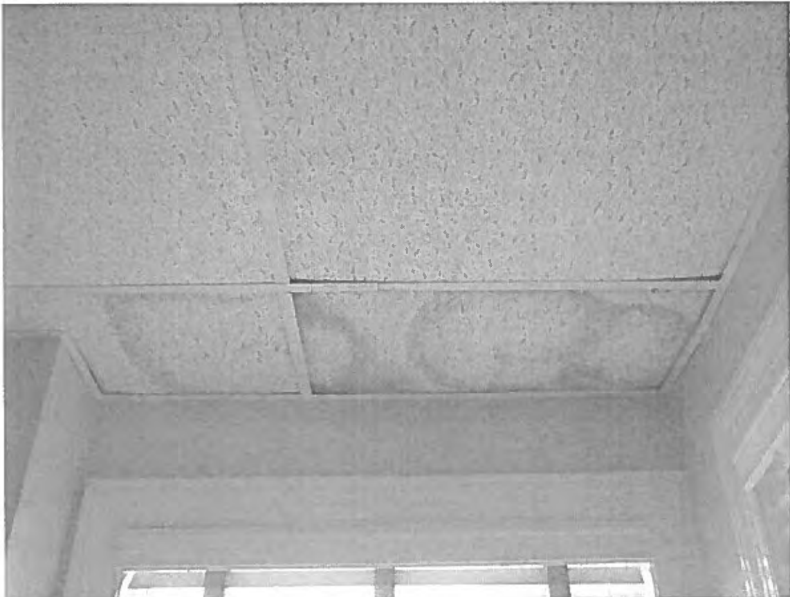
Photo 64 - Water and moisture infiltration affecting finishes
