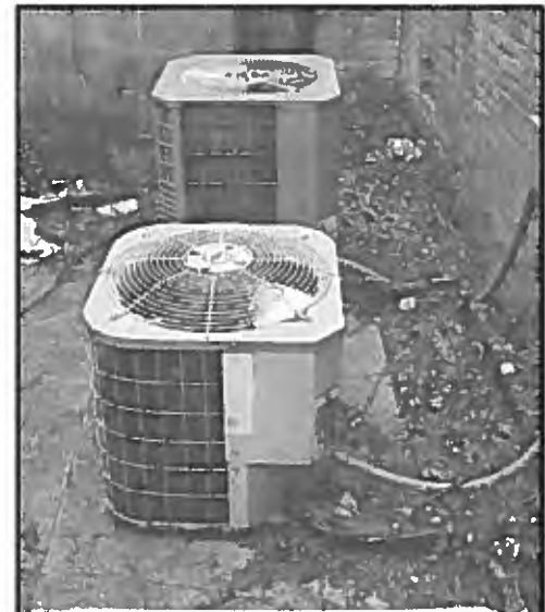
Photograph #6: Existing Condensing Units
