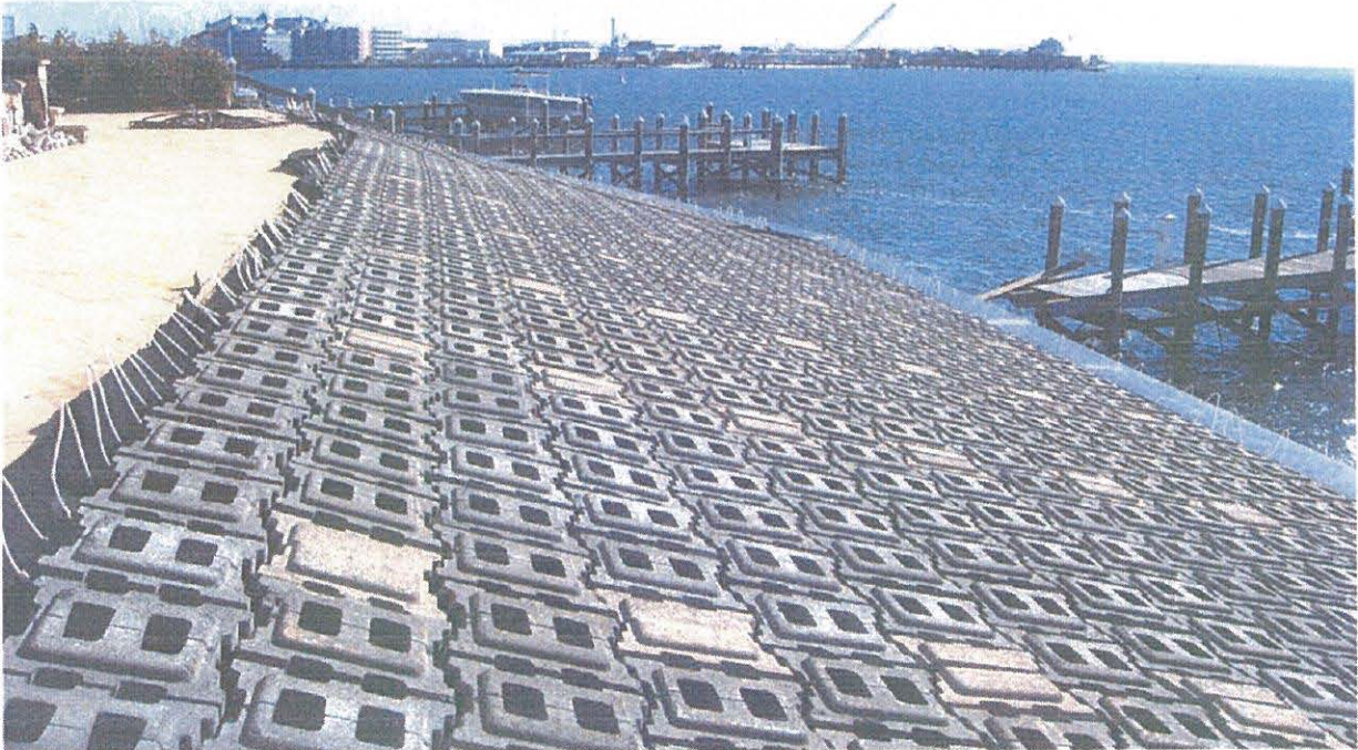
Photo showing the mats installed behind the steel bulkhead; the mats will receive plantings this season
