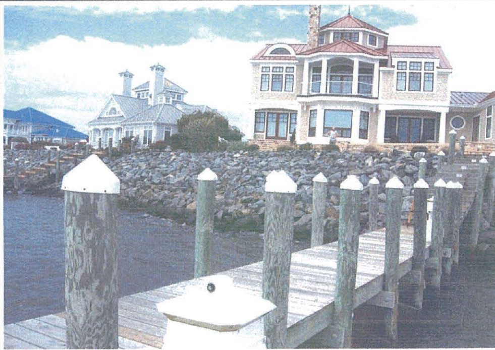
BEFORE: Photo's of the rip rap, showing the slope failure
